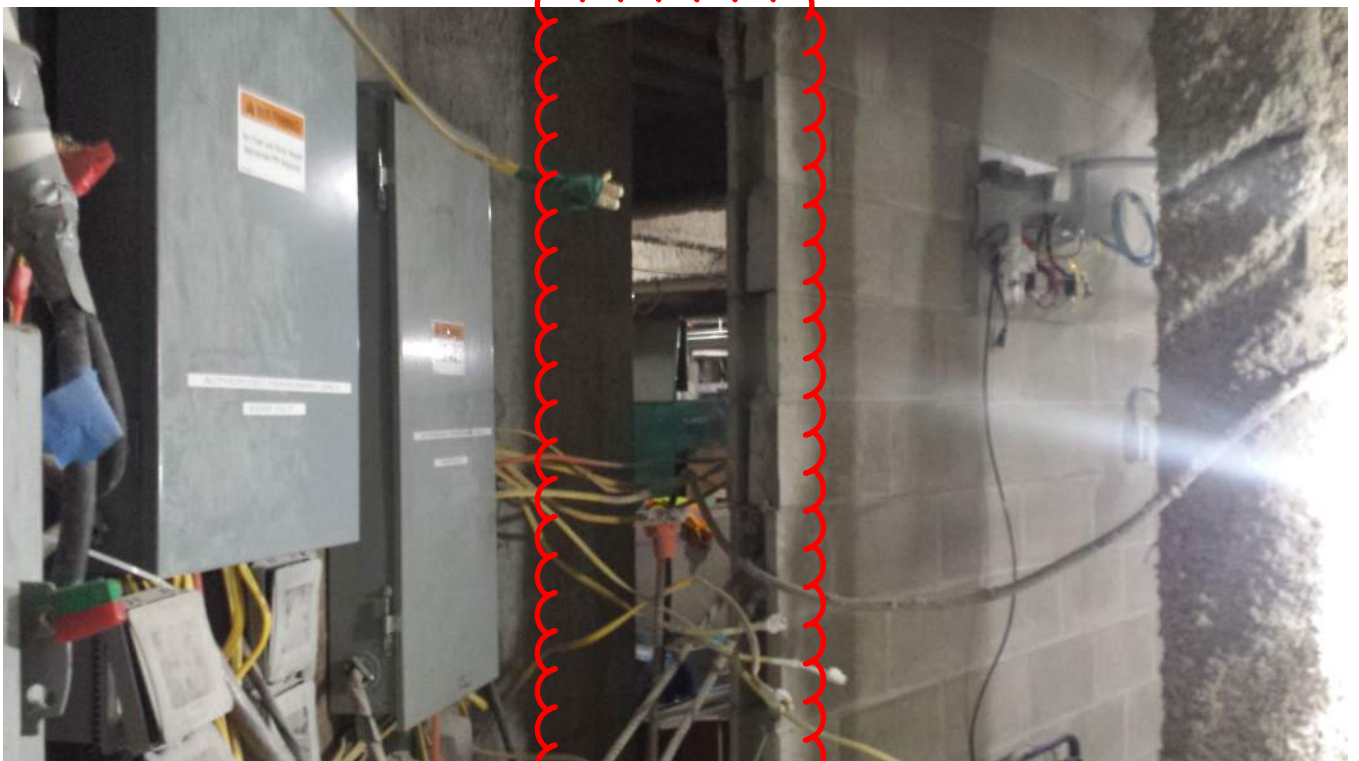
See note 23.08. Board Room 1006 shown.
