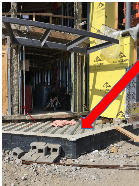
Location of Foundation damage at the intersection of A and E Lines
