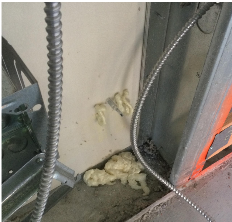
Brick tie penetrations @ Unit 1309 - Remove all brick ties that miss the stud and repair the A/V barrier per the Project Specifications
