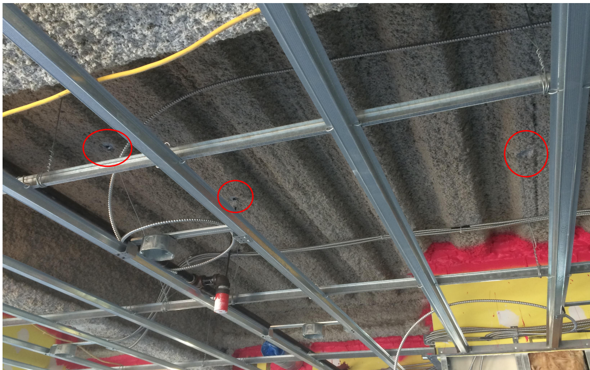
Touch up areas of spray fireproofing that have been removed for installation of new work prior to closing up the ceilings
