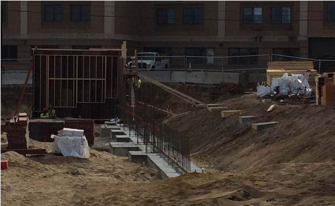
CIP footing placement along H-Line. Wall formwork along 11.2-Line visible in background
