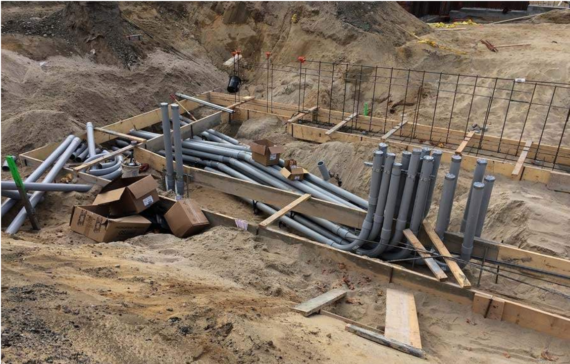
Electrical ductbank at Main Electrical Room G013
