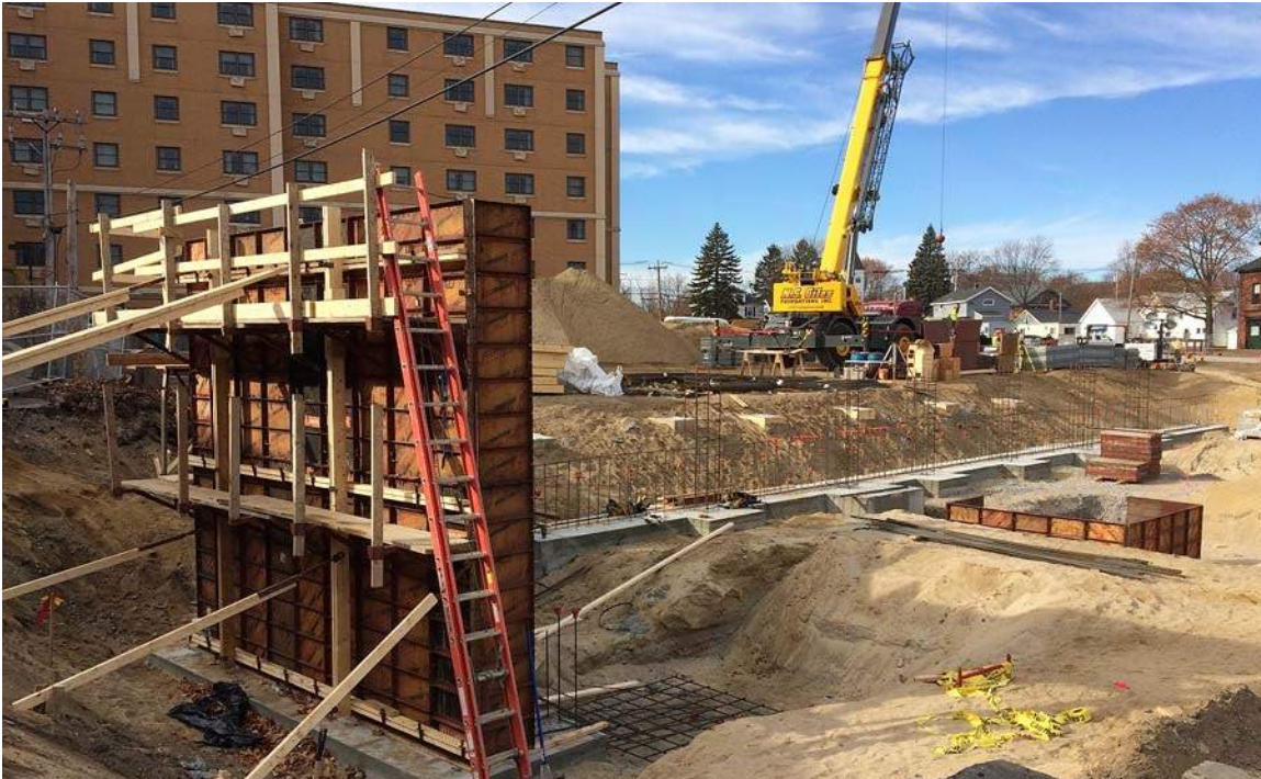
Foundation wall formwork @ 11.2-Line from G to H-Line. H-Line footings visible in the background.
