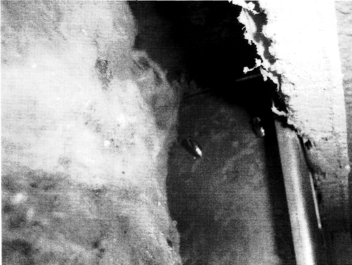
Photo 1: no visual damage to wall framing components at the 5 th floor unit
