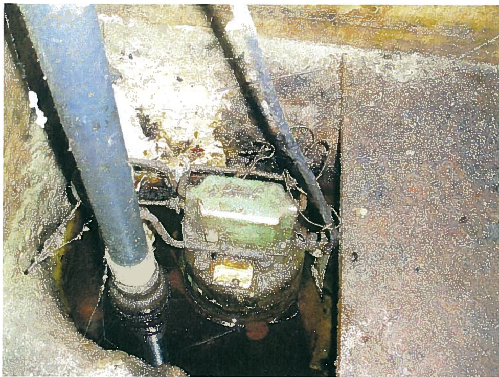
Photograph 6. Sump pump in roughly cut sump pit in southeast corner of elevator pit, looking down (south).
