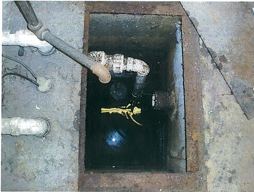
Photograph 11. Sewer ejector pit with steel plate removed, looking down (south). Top of sump pump visible with 2-in. diameter PVC effluent pipe, extending through portion of steel plate still in place.
