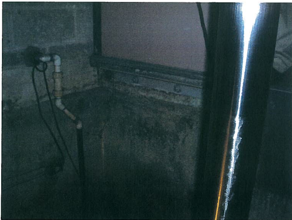
Photograph 4. Southeast corner of elevator pit, looking southeast. PVC piping from sump pump is approx. 1.25-in. OD. Sump pump is plugged into outlet shown.
