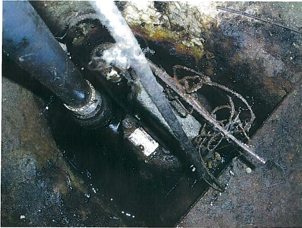
Photograph 5. Sump pump in roughly cut sump pit in southeast corner of elevator pit, looking down (southeast). Bottom of sump pit is 0.9 ft below top of elevator slab (El. 111.3), water level is 0.5 ft below top of slab (El. 111.7). Water apparently contains antifreeze.
