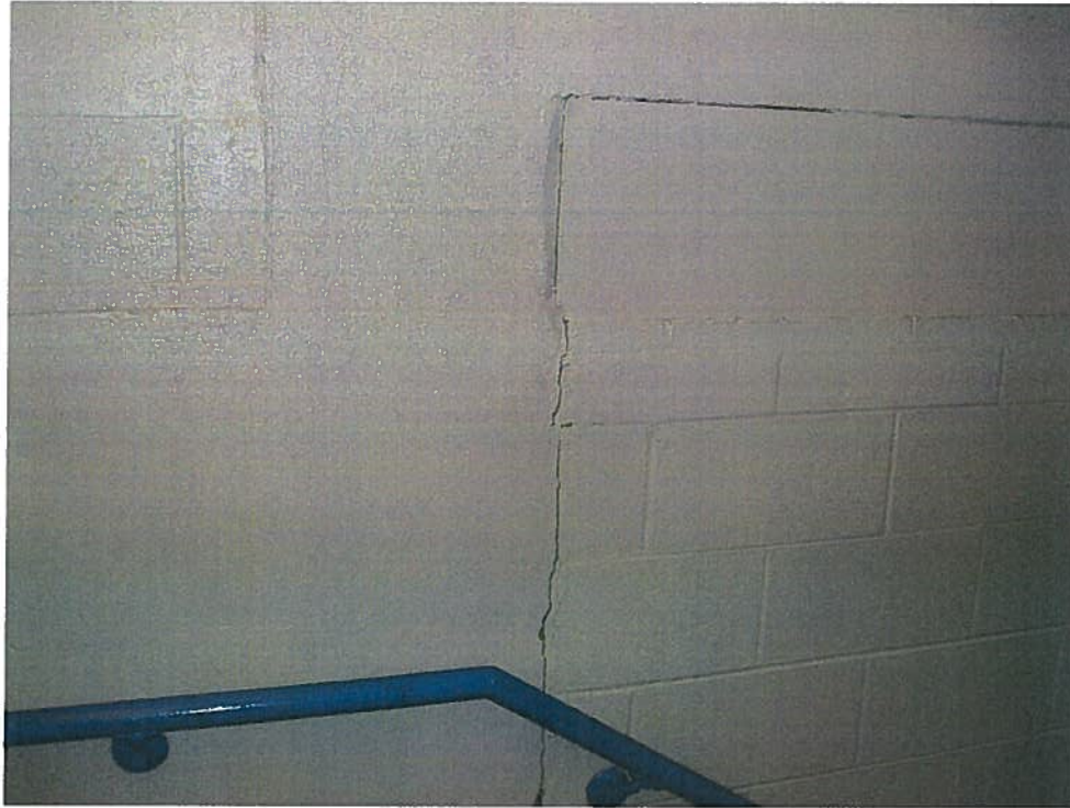
Photograph 13. Crack observed between CMU and cast-in-place concrete on east side of stairway wall, looking east. Maximum crack opening width was approximately 3/32 in. wide.
