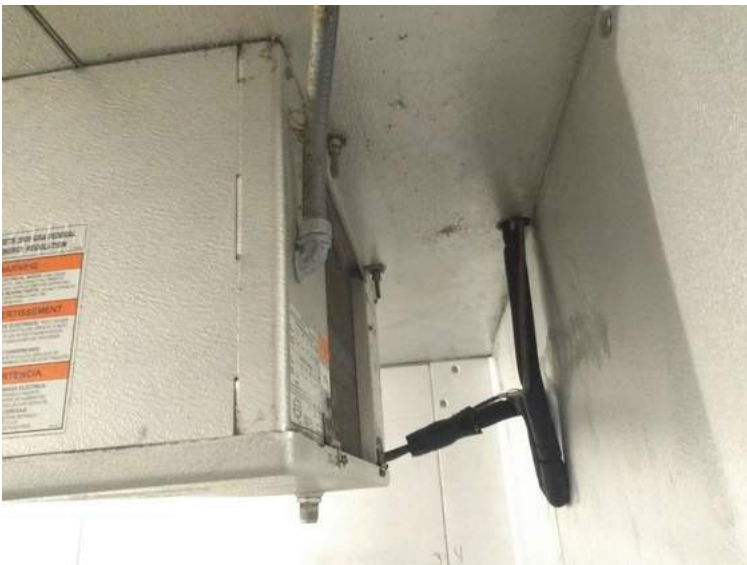
Back of Cooling Unit
