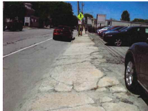
Southern curb cut apron (to be narrowed and repaired)
