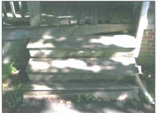
2.4 Picture 8 Stairs at rear porch need replacing
