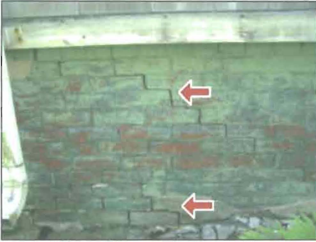
2.7 Picture 1 Step cracks show settlement
