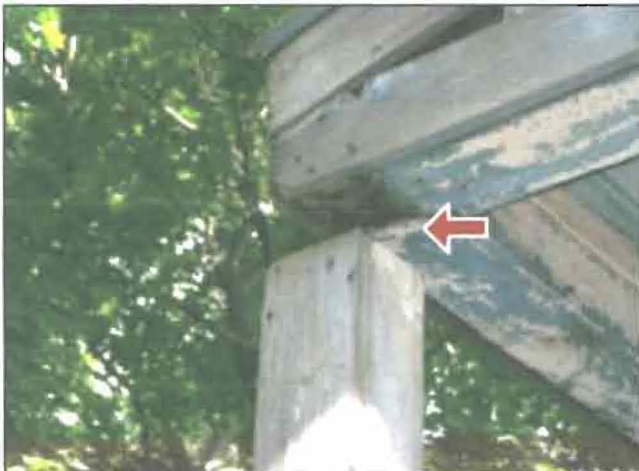
2.4 Picture 7 Column detached at rear porch
