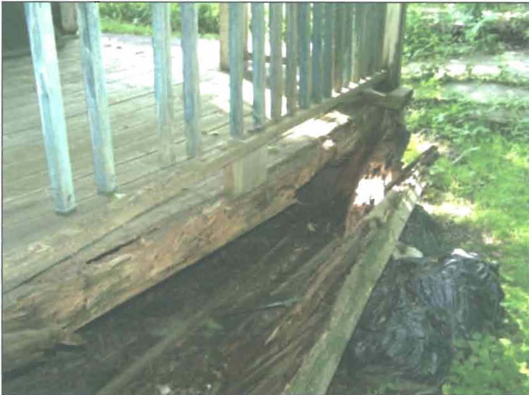
2.4 Picture 6 Rear deck is a total
