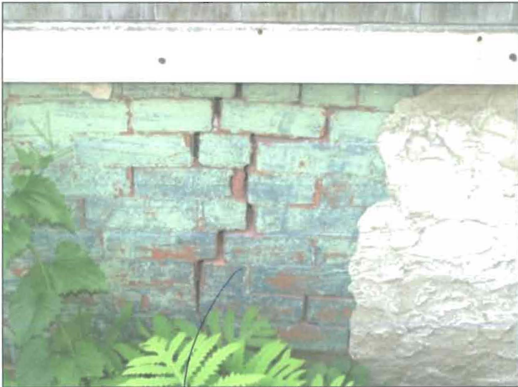
2.7 Picture 3 Step crack at right side, rear
