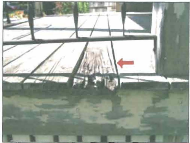
2.4 Picture 5 Bad decking on front porch
