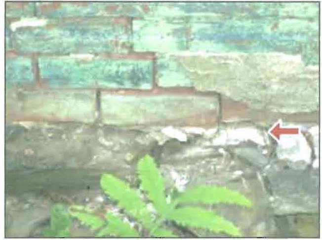
2.7 Picture 2 Pointing needed in various areas
