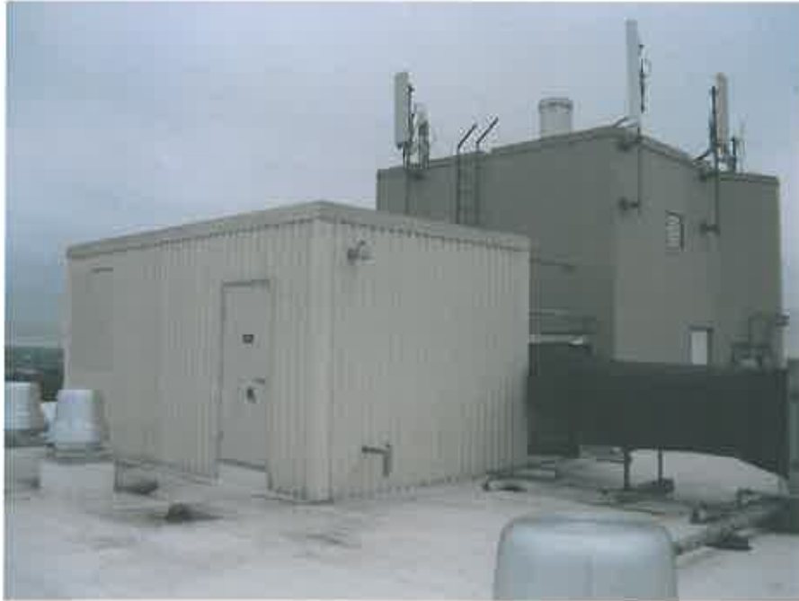
Photo 1: Sample photo illustrating the existing equipment shelter.
