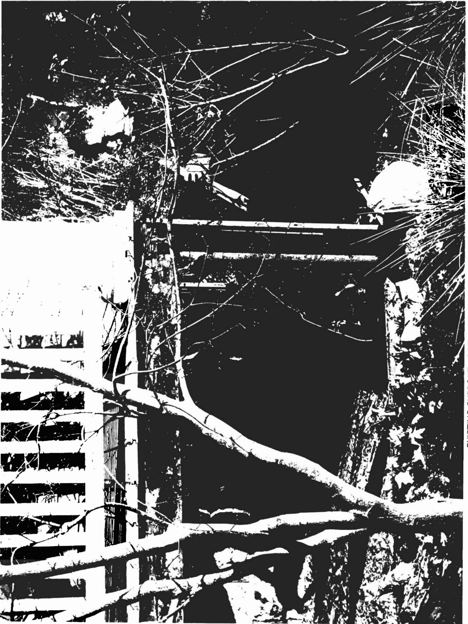
EXISTING SUPPORT POST - RUSTED 3" PIPE SET ON BRICKS.JPG
