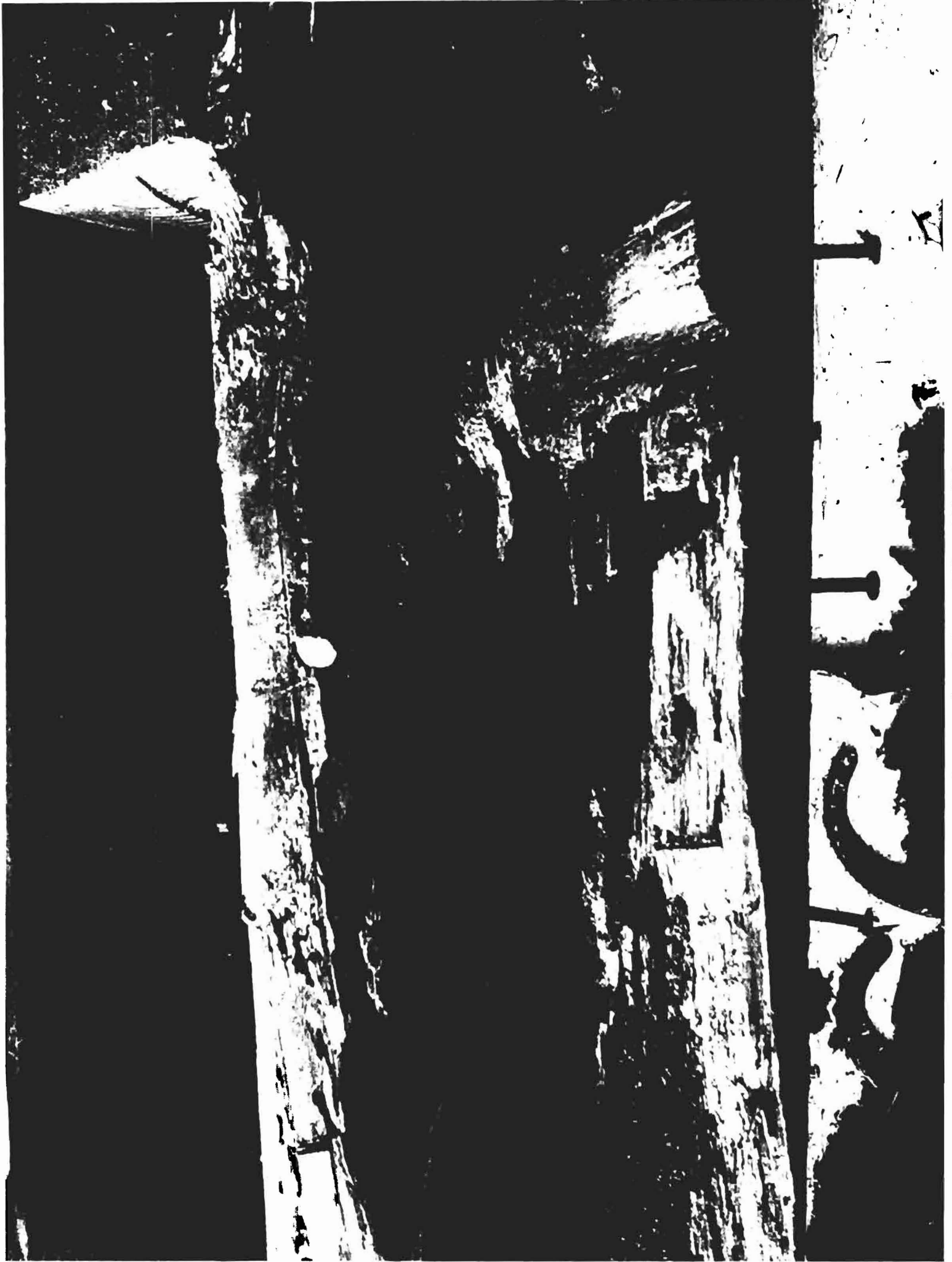
ROT IN EXISTING CARRYING BEAM.JPG
