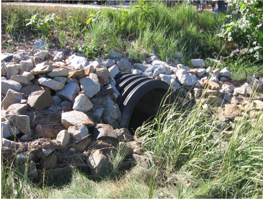
Image 3: Looking Northwest at the existing 36" outfall pipe (taken by Gary Fullerton on 9/16/16).
