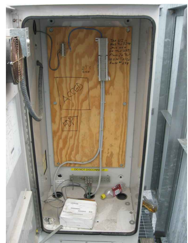
EXISTING TELCO CABINET ④ T-2
