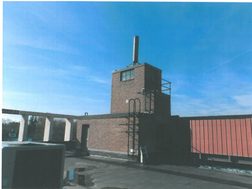
Photo 2: Sample photo showing the existing ballasted canister to be removed and replaced.
