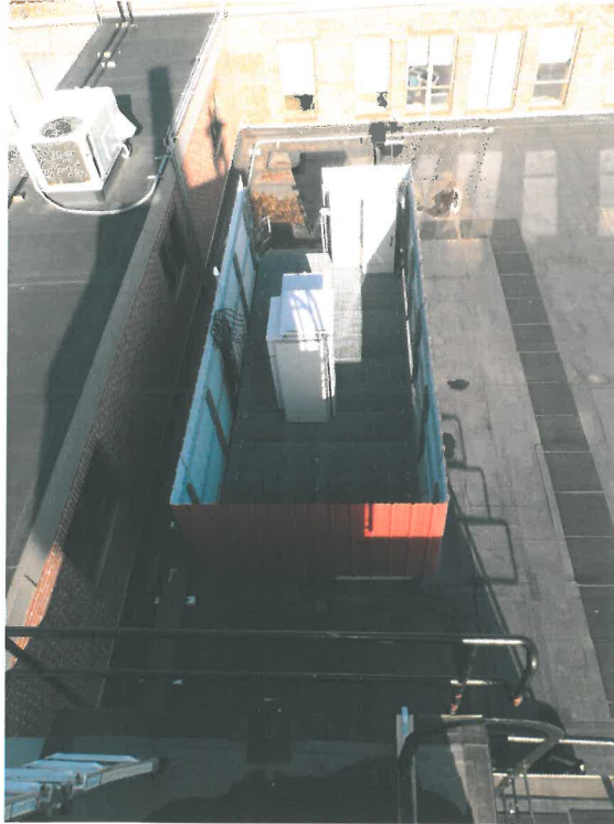
Photo 4: Sample photo showing the existing Sprint equipment platform.
