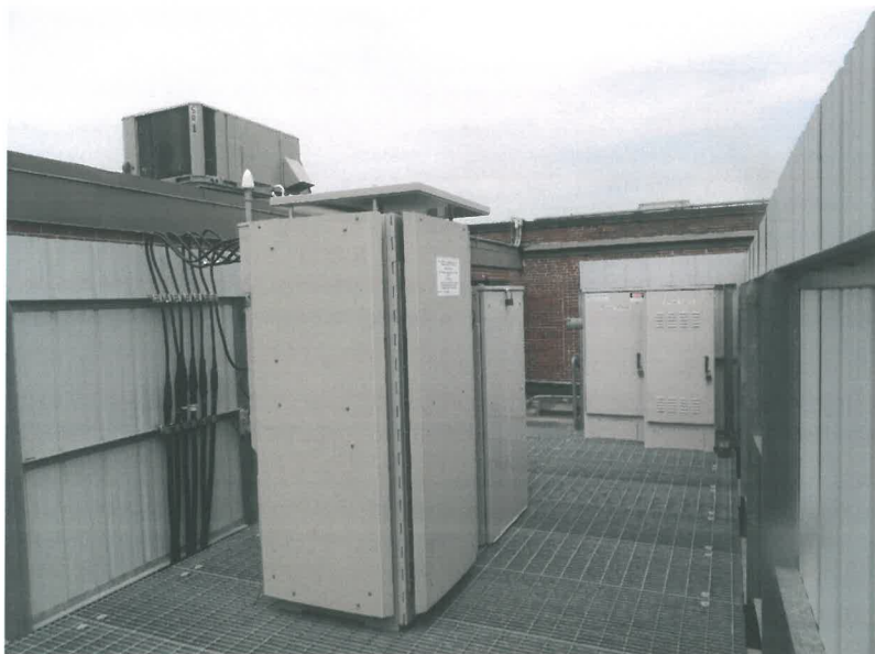
Photo 5: Sample photo showing the existing Sprint equipment.
