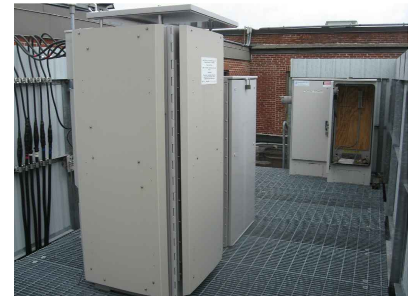
EXISTING EQUIPMENT AREA ③ T-2
