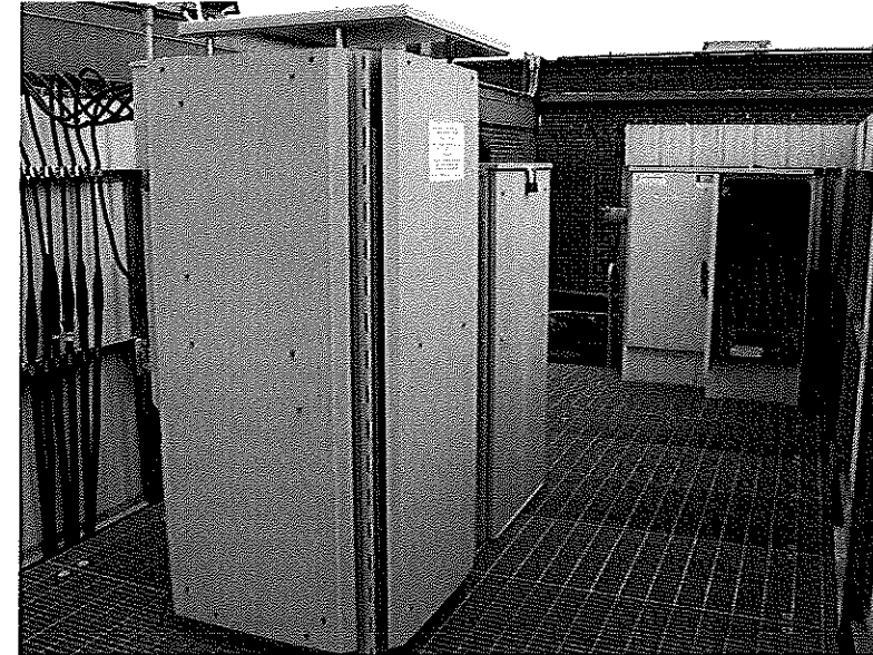
EXISTING EQUIPMENT AREA 3 T-2
