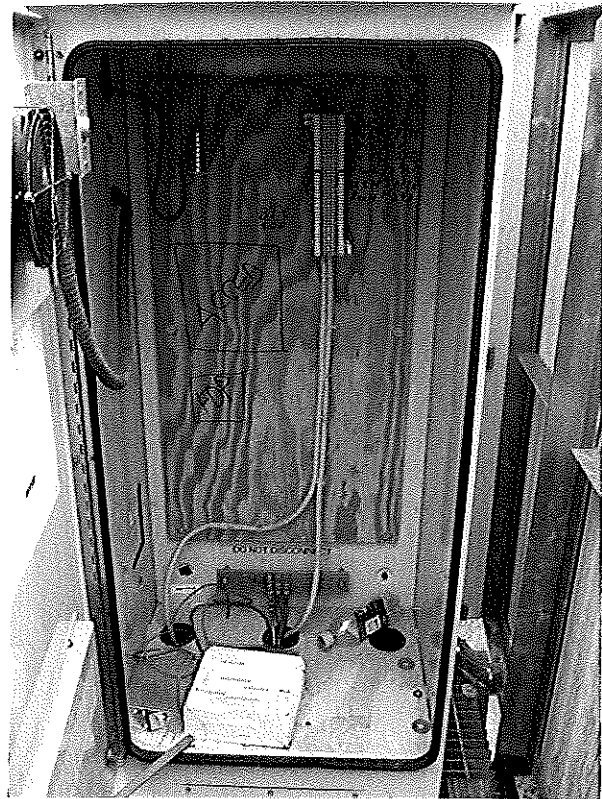
EXISTING TELCO CABINET 4 T-2
