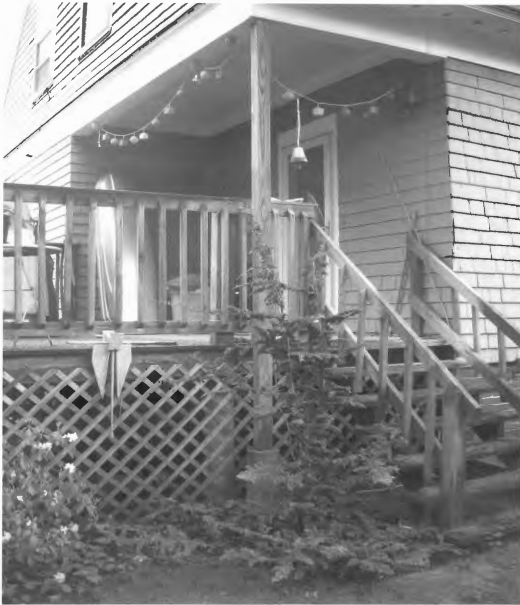
Porch to be removed, footer installed and space framed in. New porch within dimensions of old deck.
