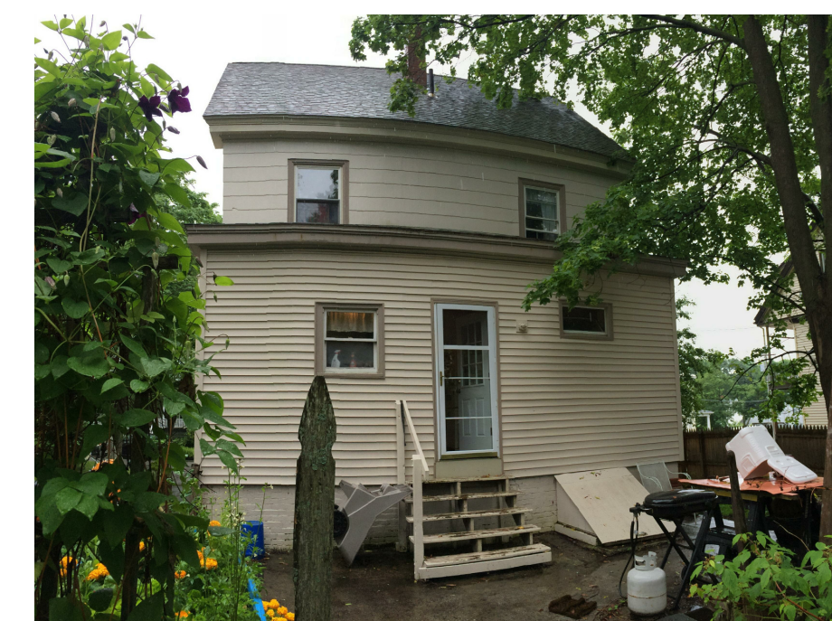
EXISTING EXTERIOR FACADE. NOTE FIRST FLOOR VINYL SIDING AND UPPER STORY ASBESTOS SHINGLES.
