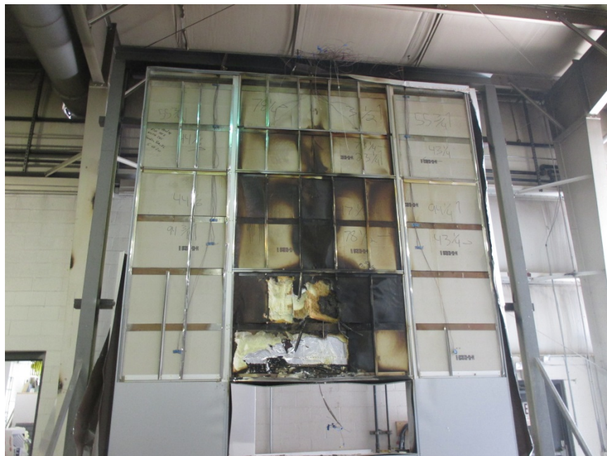
Photo No. 16 Burn Pattern of Insulation (Exterior Cladding Removed)
