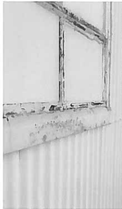
Figure 2: Asbestos window caulking
