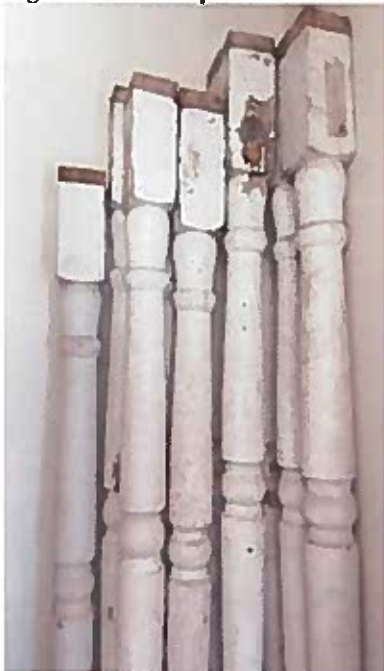
Figure 5: Lead Painted post
