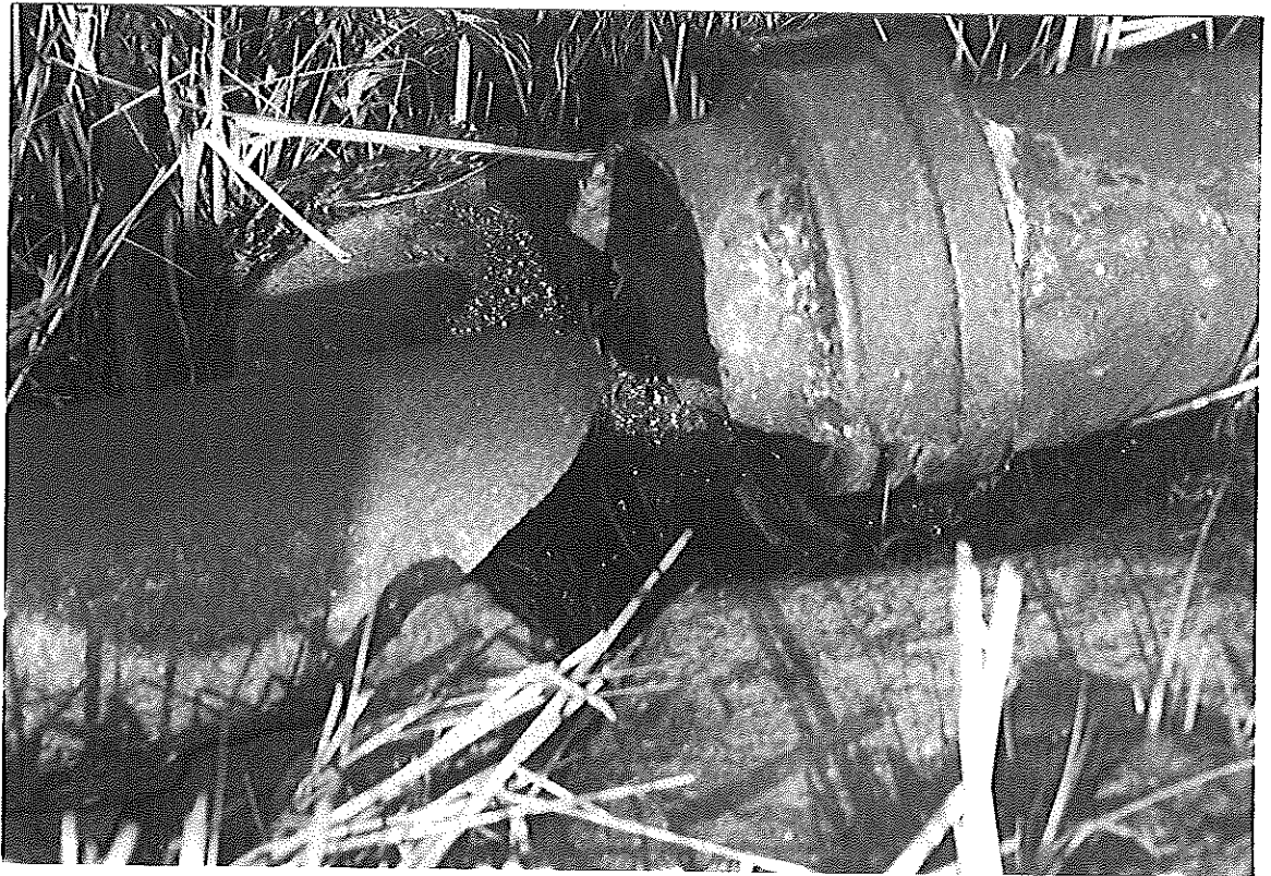
Break in pipe, but a major leak is about 10 feet before this break
