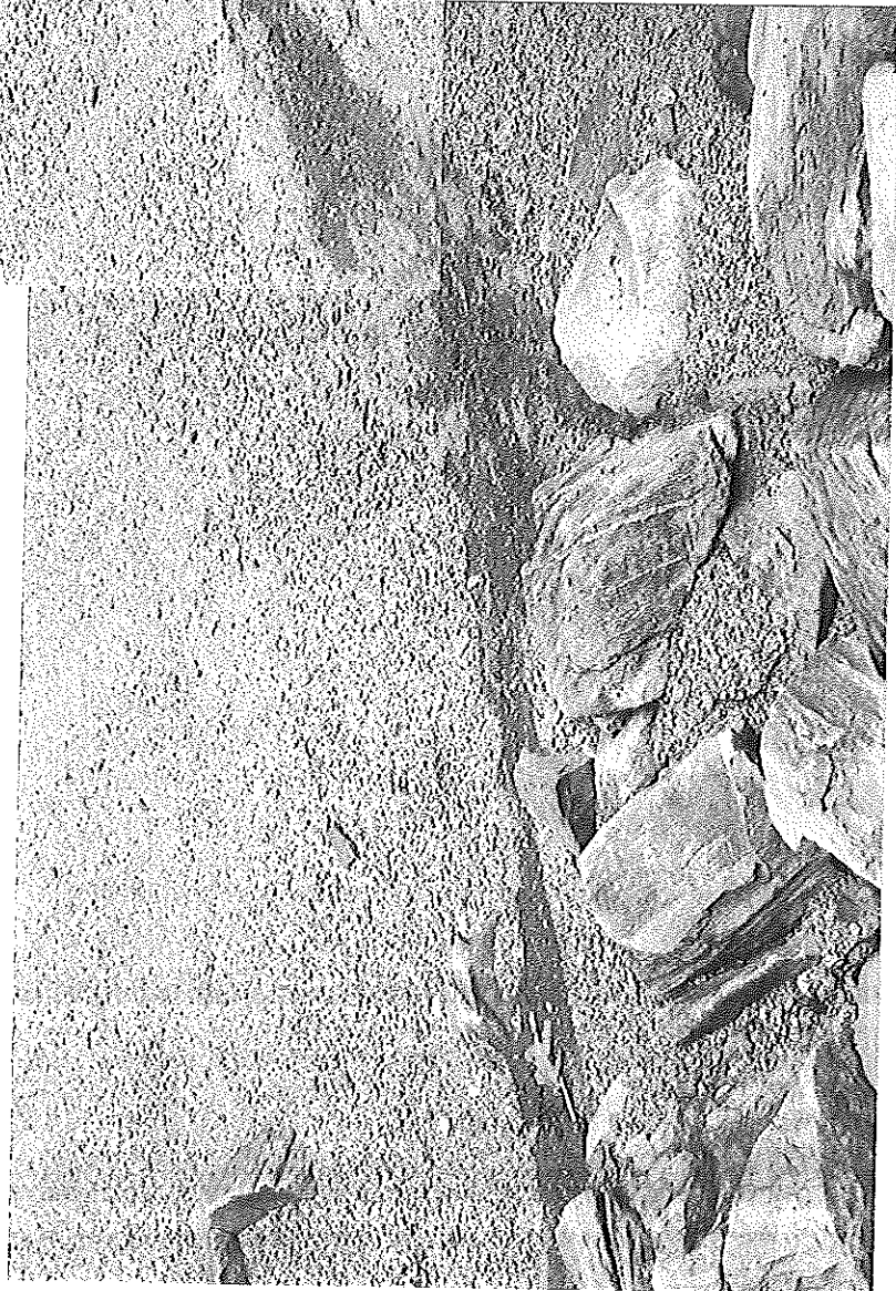
very early spring -- greasy drainage from underground leaks in sewer pipe
