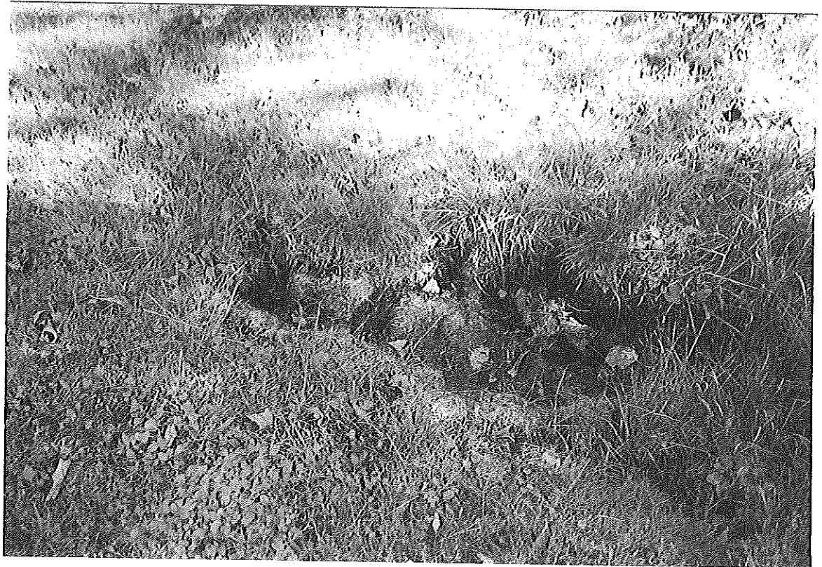
erosion from leaking sewer pipe next to large dug well
