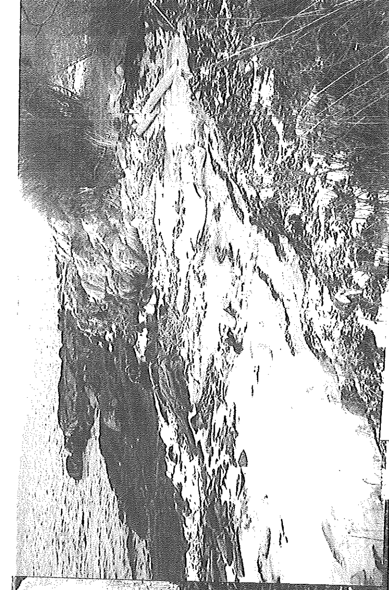
frozen drainage from leaks in pipe
