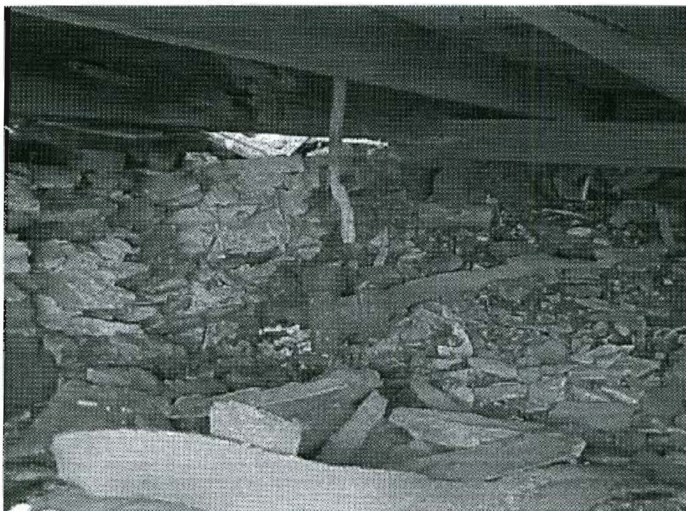
Photo 3: View of underneath existing dwelling with remains of lead pipe and cast iron drain pipe.
