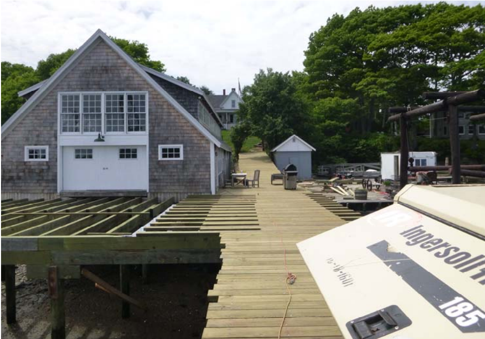
Figure 5. View of pier building from front. Pier construction in progress. Building support complete (Photo taken 6-11-14).
