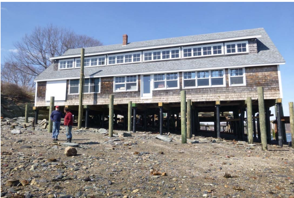
Figure 4. View of south side of building in place on new support piles and caps. Pier construction in progress (Photo taken 4-11-14)
