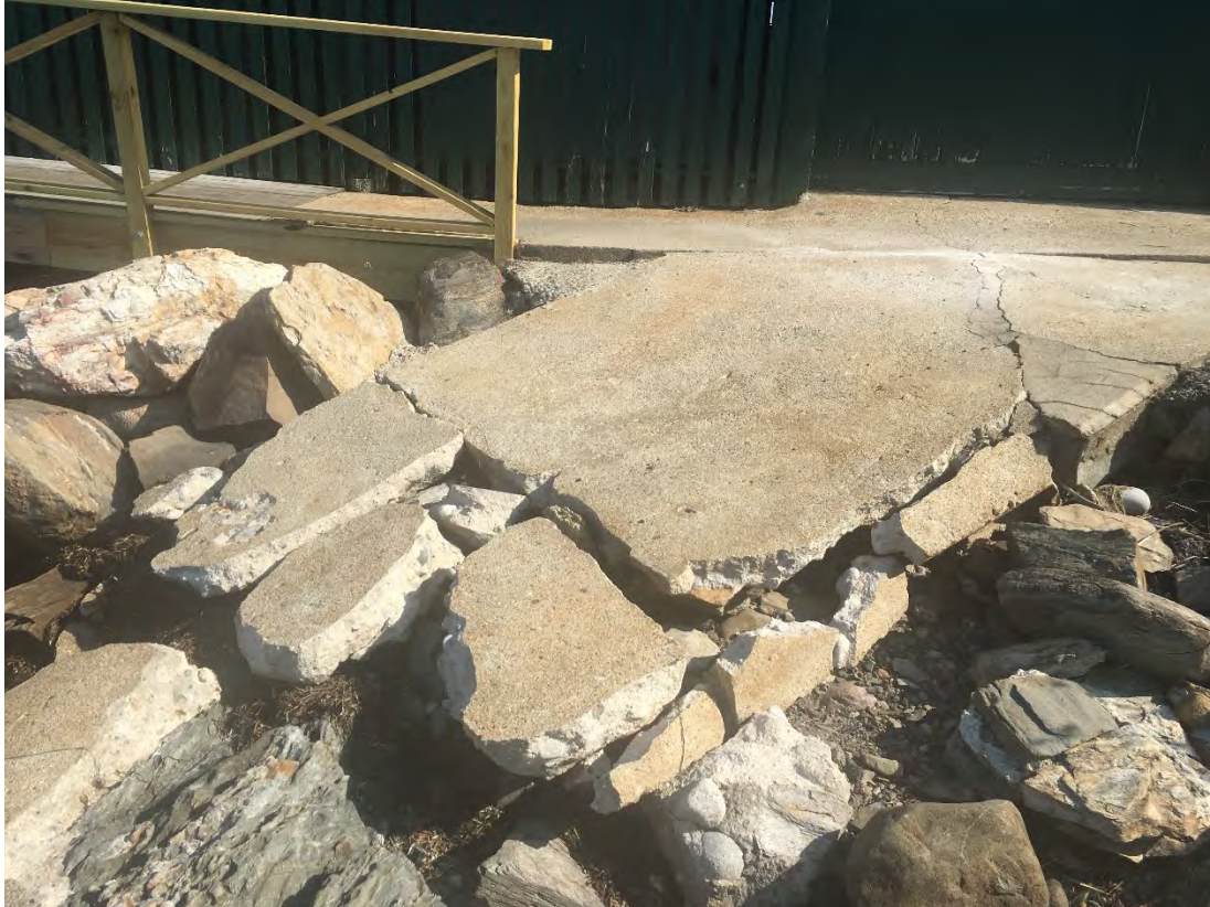
View of Erosion of Boat Ramp (looking northeast)
