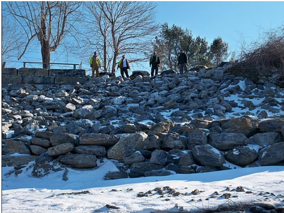
Boulder Shoreline Stabilization in the Vicinity of 29 Oaklawn Rd., Peaks Island (Photo by William R. Walsh, WEA, February, 2011)
