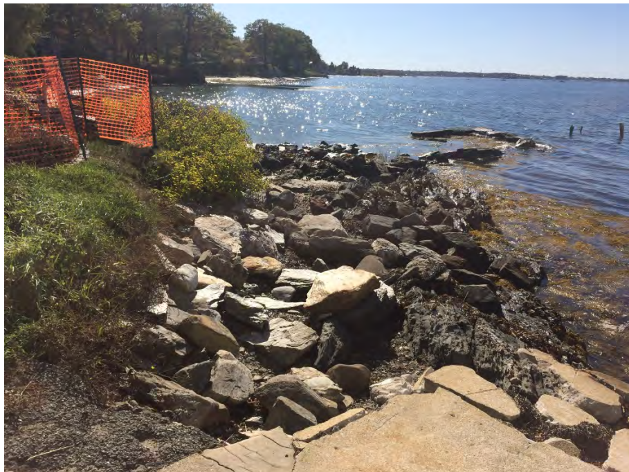
Photo 2: View of eroded bank looking south (Photo by Silas Canavan, WEA, October 2017)
