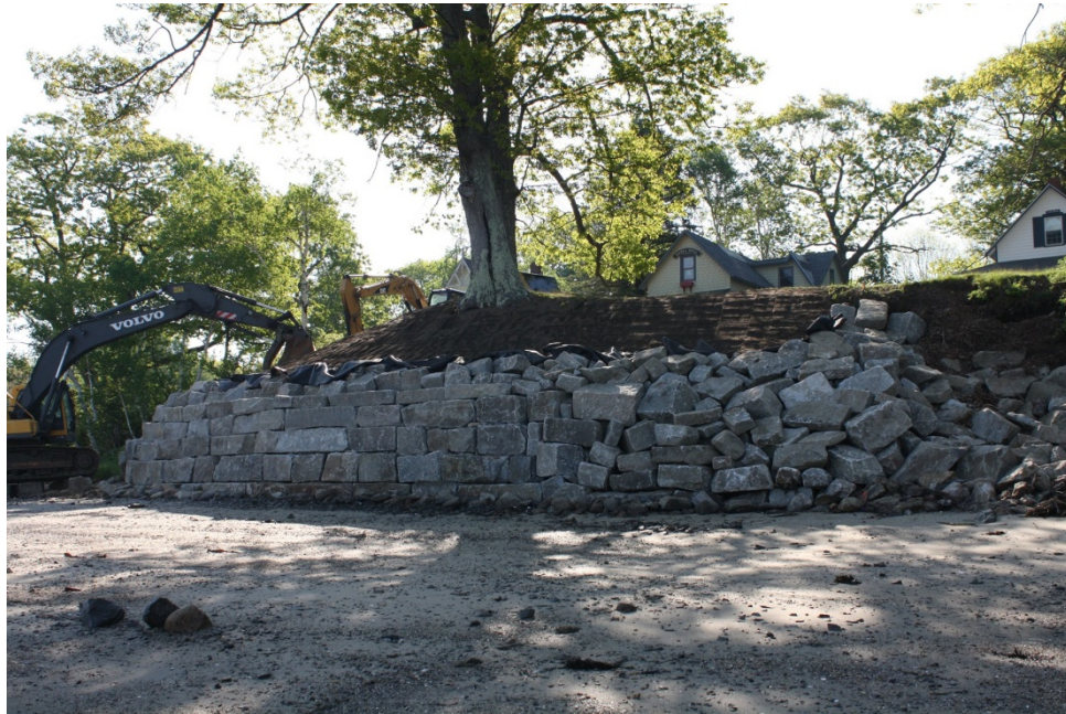
View of Existing Seawall at to 35/39 Oaklawn Road, Peaks Island (Photo by William R. Walsh, WEA, May 2013)
