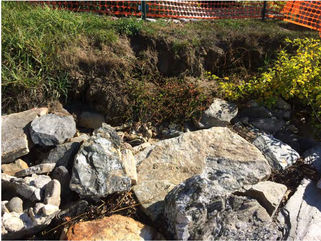
View of Erosion of Existing Embankment (looking east)
