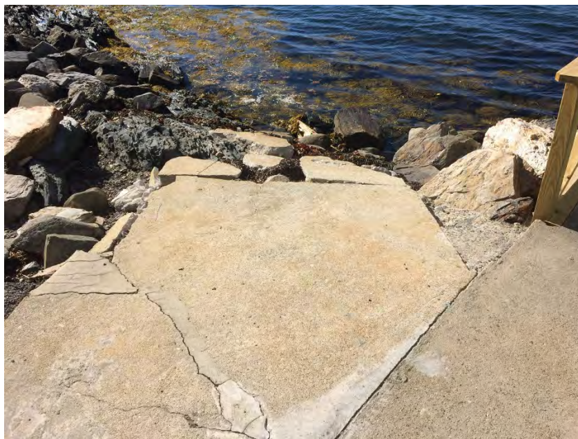
Photo 4: View of deteriorated boat ramp looking west (Photo by Silas Canavan, WEA, October 2017)
