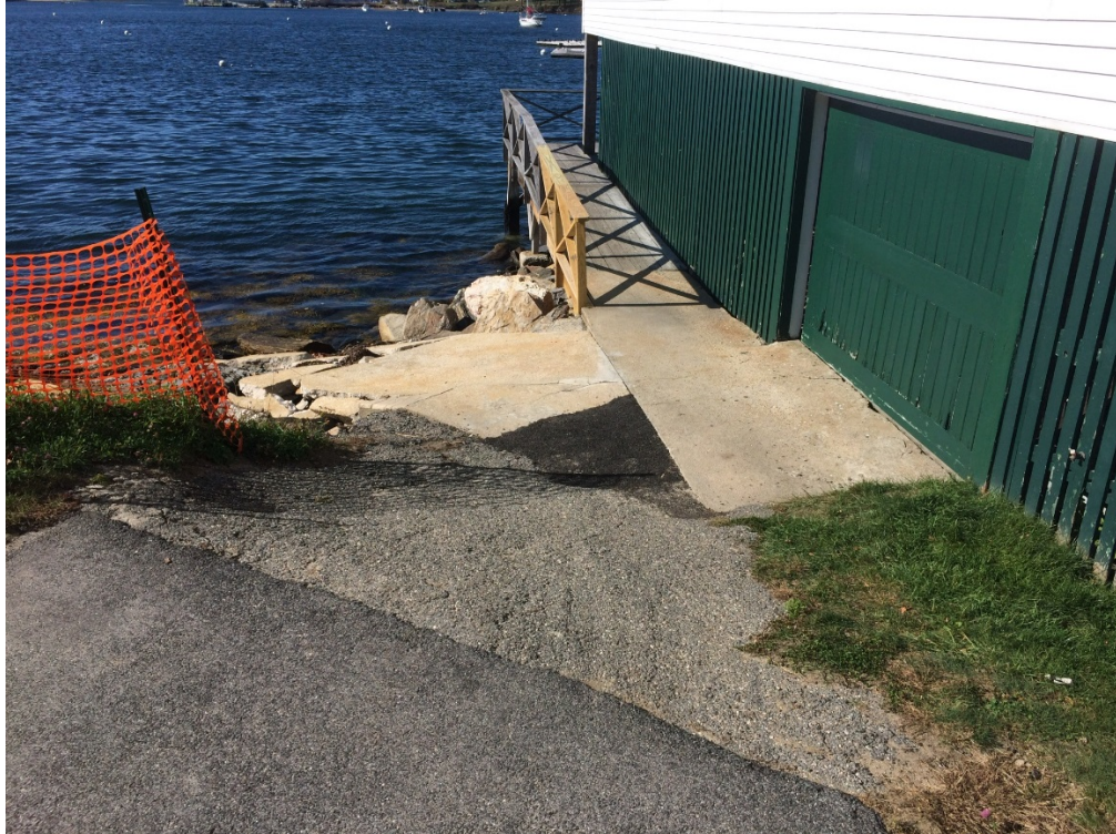
View of Existing Boat Ramp at 10 Trefethen Avenue, Peaks Island, ME (Photo by Silas Canavan, WEA, October 2017)
