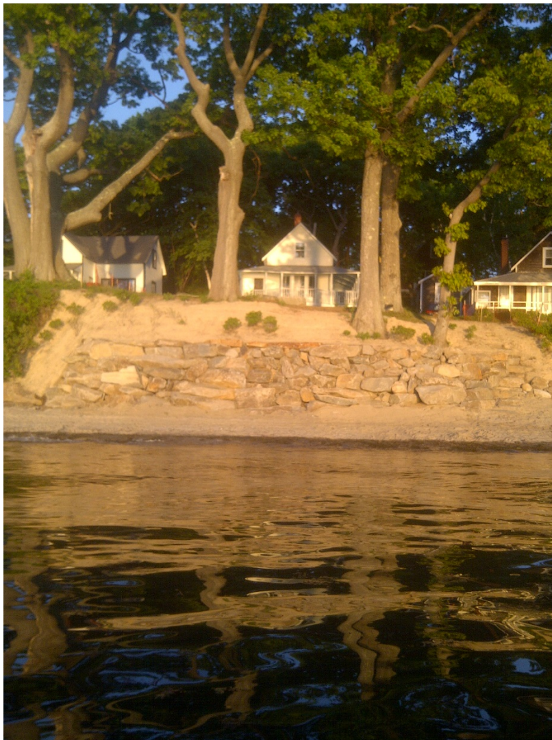
View of Existing Sea Walls at 29 Oaklawn Road, Peaks Island (Photo by Silas Canavan, June 2016)
