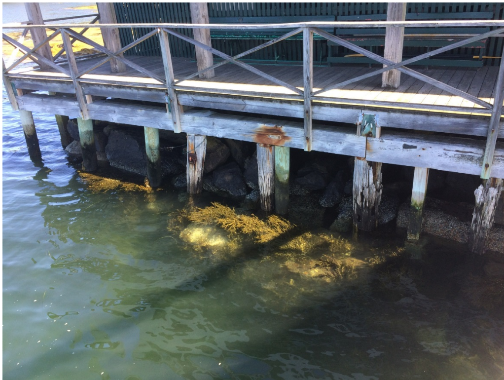
View of Existing Deck Piers at 10 Trefethen Avenue, Peaks Island, ME (Photo by Silas Canavan, WEA, October 2017)
