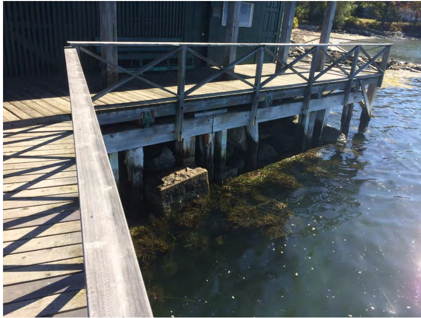
Photo 5: View of western-facing deck piers to be protected (Photo by Silas Canavan, WEA, October 2017)
