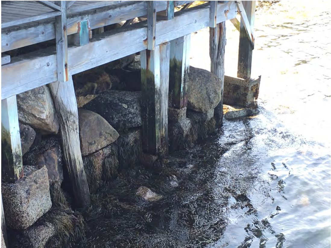
View of Erosion of Deck Piers (looking southeast)
