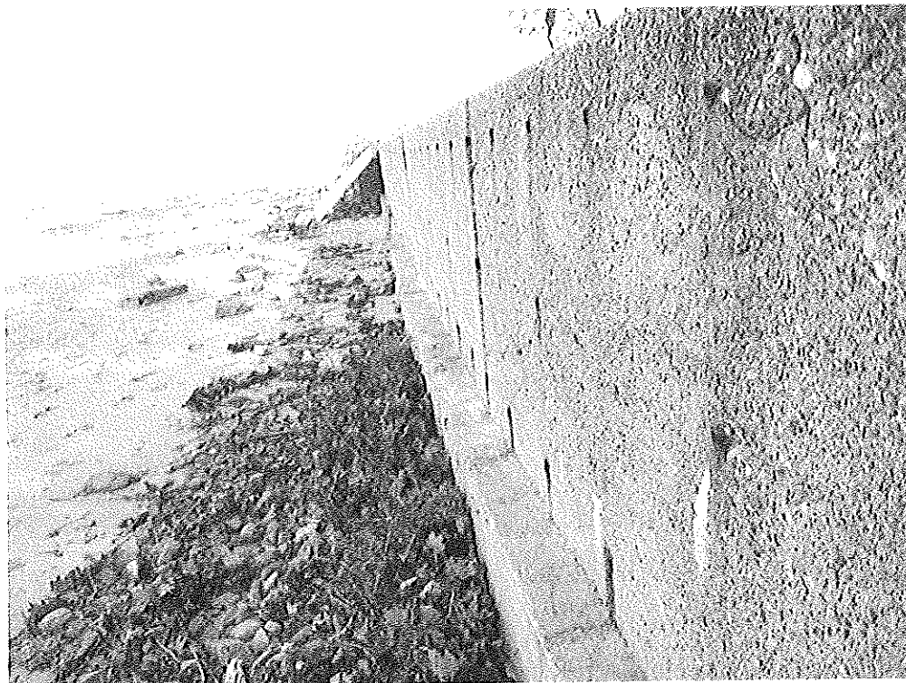
Detail photo of existing seawall (Photo by William R. Walsh, WEA, November, 2010.)
