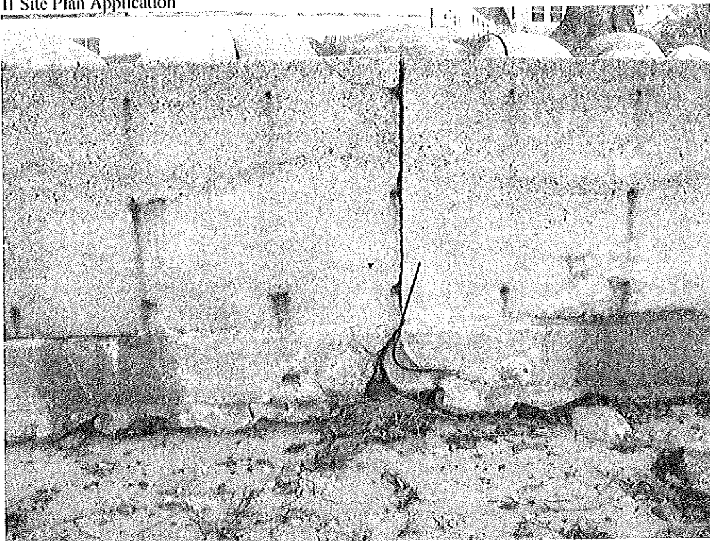
Detail photo of existing seawall showing undermined foundation. Photo by William R. Walsh, WEA, November, 2010.
