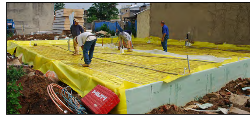
AIR SEALING AT WALLS: LEAVE VB LONG, TO ALLOW FOR TAPE SEAL TO WALL SHEATHING AFTER FRAMING
