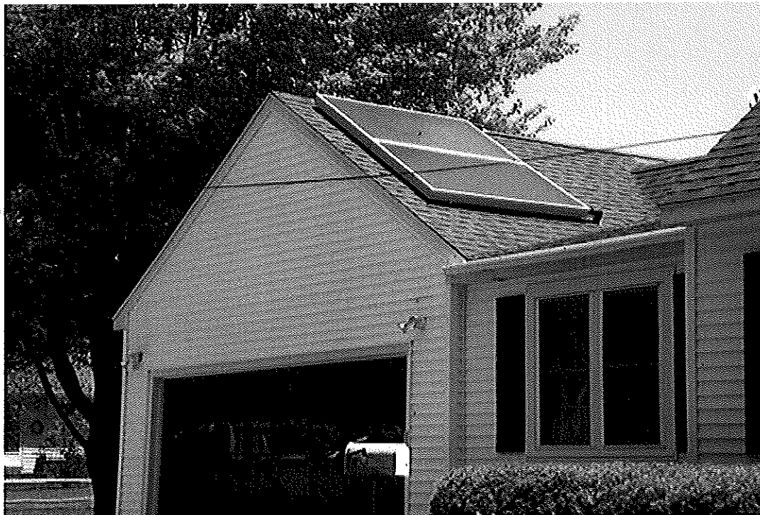
Above are two flat plate solar hot water collectors installed by ReVision Energy. This is the type of flush mount installation we are proposing for your home.
