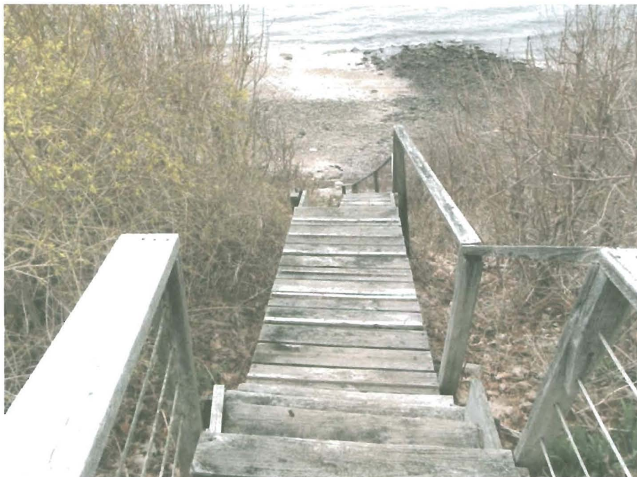
View of existing stair from lawn. Vegetation clearing required 2 ft either side of stair for new construction.
