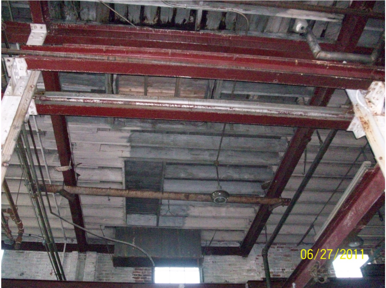
Peaks Island Low roof north portion penetration to be removed and roof requiring reframing.
