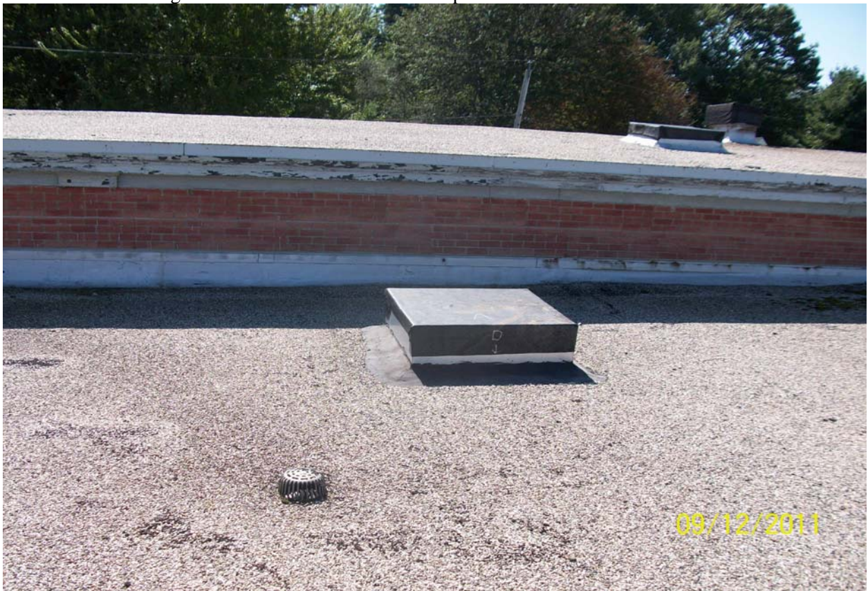
Peaks Island Building. Lower roof to be reroofed. All penetrations to be removed. One of the existing two (2) roof drains that will be replaced.
