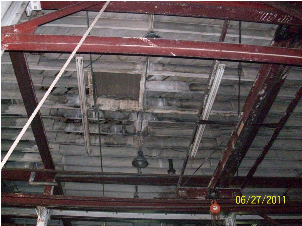
Peaks Island Low roof portion requiring reroofing framing and new decking.
