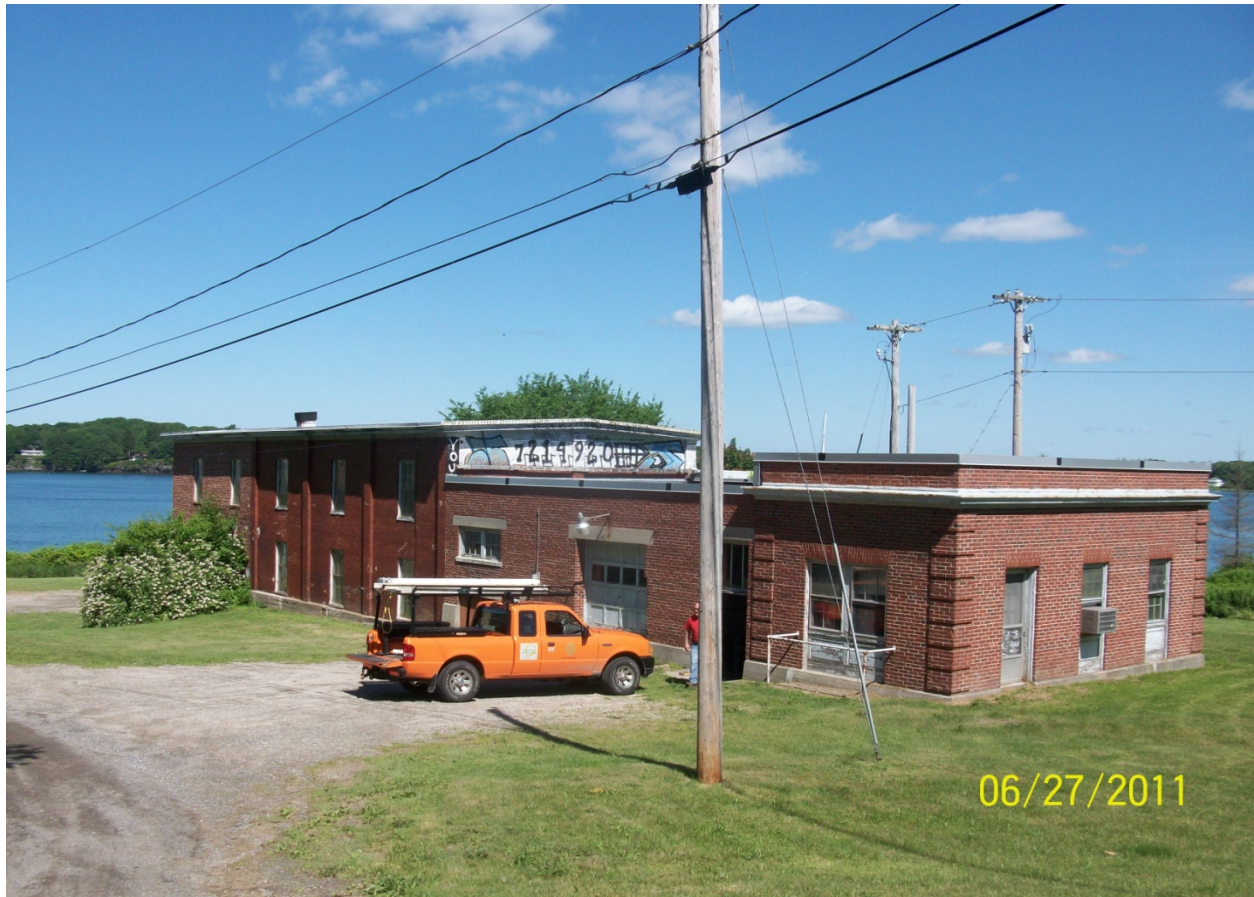
Peaks Island Building. South Elevation. Office in foreground, High roof (bay) to rear left and low roof (bay) to rear right. Office door to be replaced is behind the person in red.
