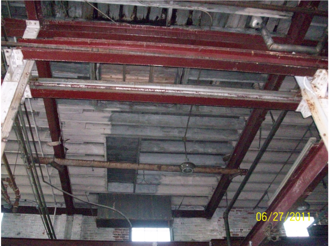
Peaks Island Low roof north portion penetration to be removed and roof requiring reframing.
