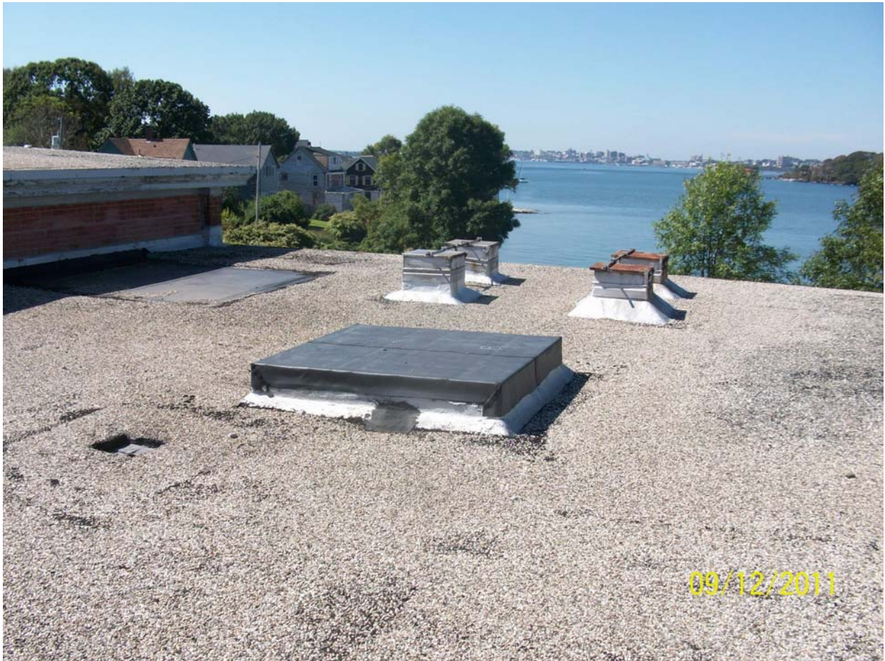
Peaks Island Building. Lower roof to be reroofed. All penetrations to be removed.
