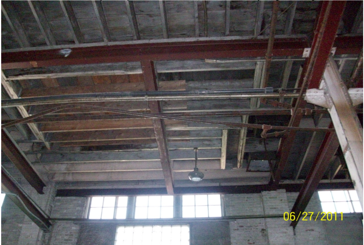
Peaks Island Low roof west portion to require reframing.
