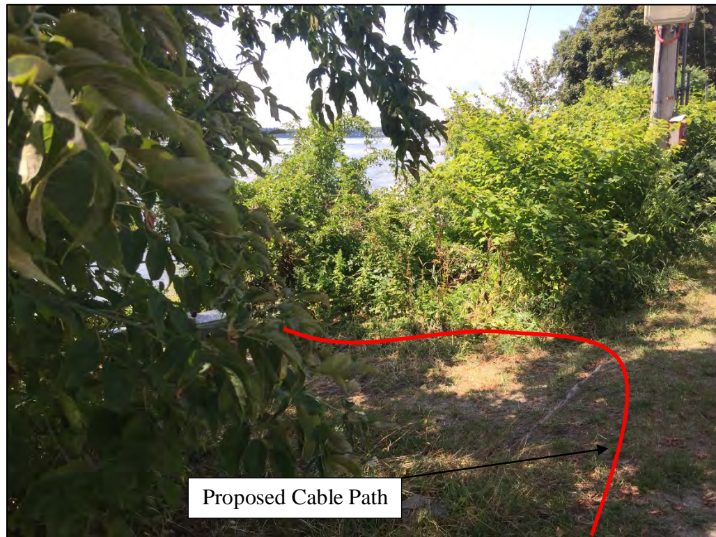
Photo 2. Peaks Island facing west towards existing riser pole. Cable will be buried along the slope, towards the beach.
