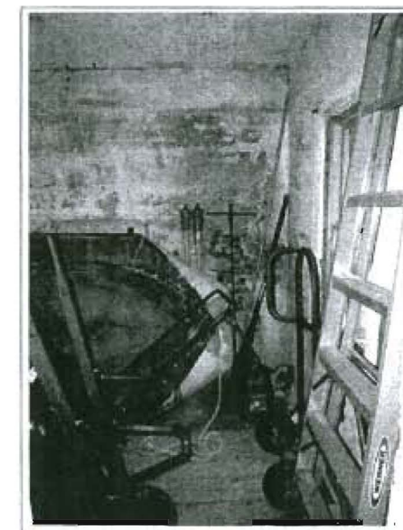
INTERIOR - STORAGE BATTERY ROOM
