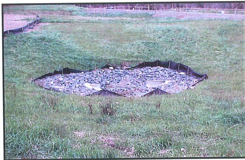
POORLY STABILIZED INLET ALLOWS ENTRANCE OF DEBRIS AND REDUCED CAPACITY
