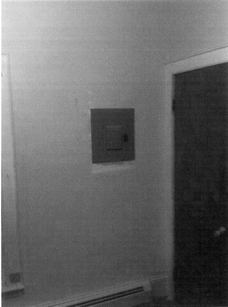
12 2 Unit Elec Panel 1 Date Taken: 2/18/2013 Taken By: ANDREW1 Electrical panel on second floor belonging to Unit 2.
