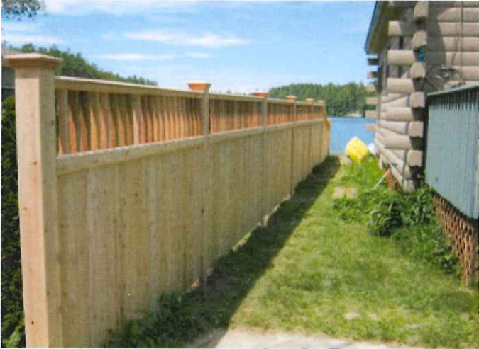
6' Board Fence with 2' Finial and a Scallop 6' to 4' Sloped Section at Street
