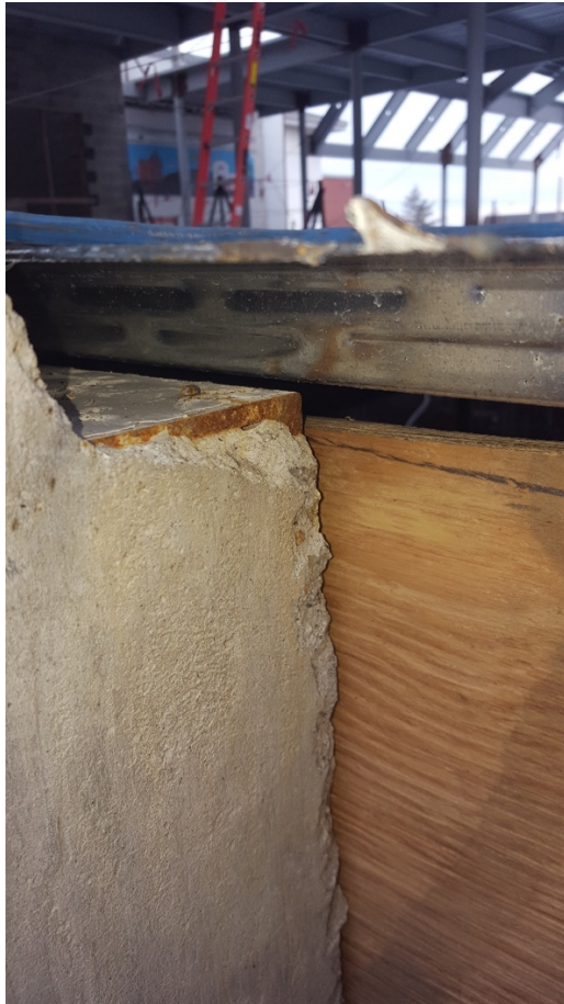
2 nd Floor deck not on/welded to the 4X4 angle
