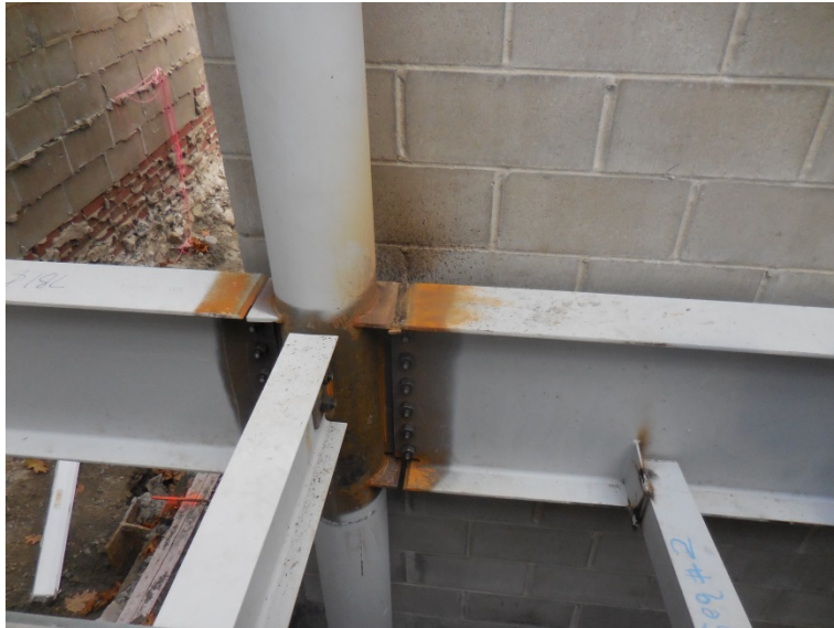
Bottom flange adjacent to CMU wall cannot be accessed for welding
