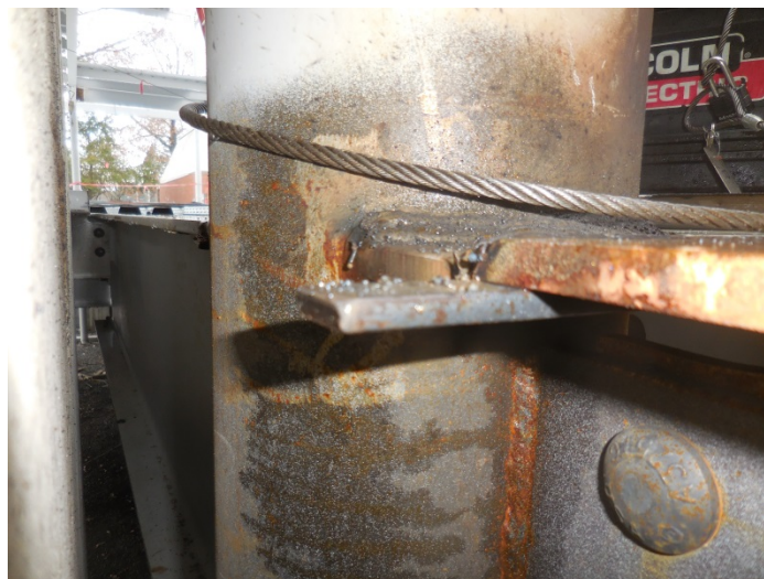
Misaligned top flange at Q/9
