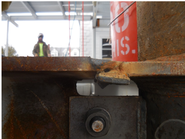
Example of 1/8 +'' misalignment at N/8
