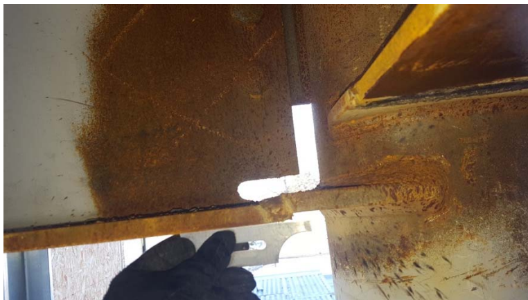
Misaligned moment connection at N/11 south
