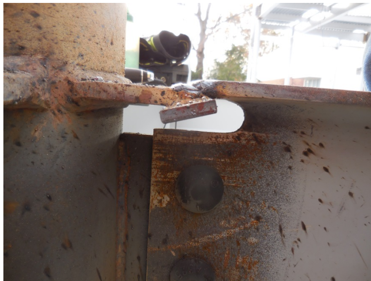
Worst case of misalignment observed (F/7 north)
