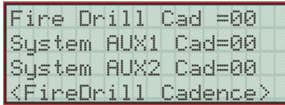
Figure 7-17 Special Cadence Patterns for Fire Drill and Auxiliary Alarm Events
