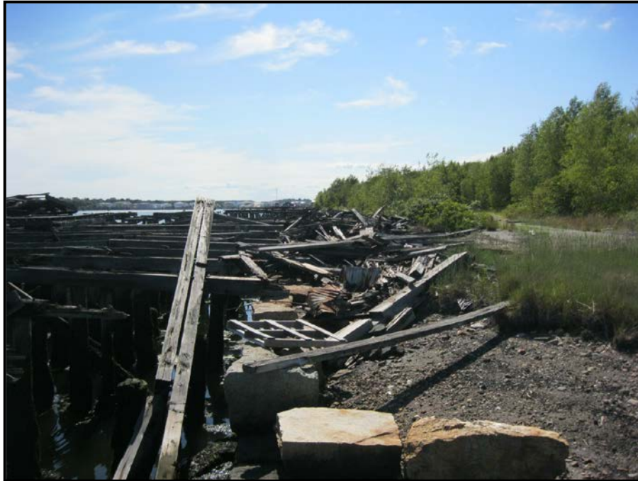
PHOTO 1 – Dilapidated Pier Remains
