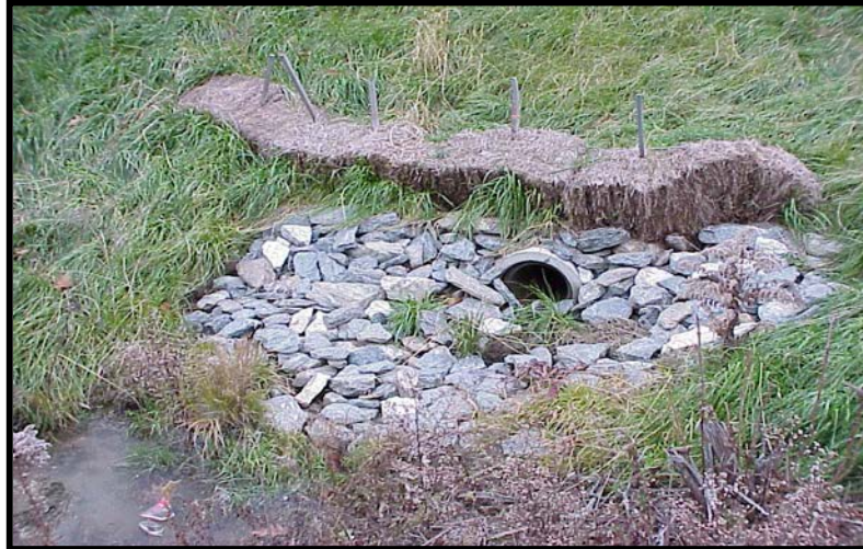
POORLY STABILIZED INLET ALLOWS ENTRANCE OF DEBRIS AND REDUCED CAPACITY
