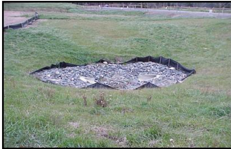
STABILIZED INLETS REDUCE DEBRIS ACCUMULATION AND MAINTAIN DESIGN CAPACITY
