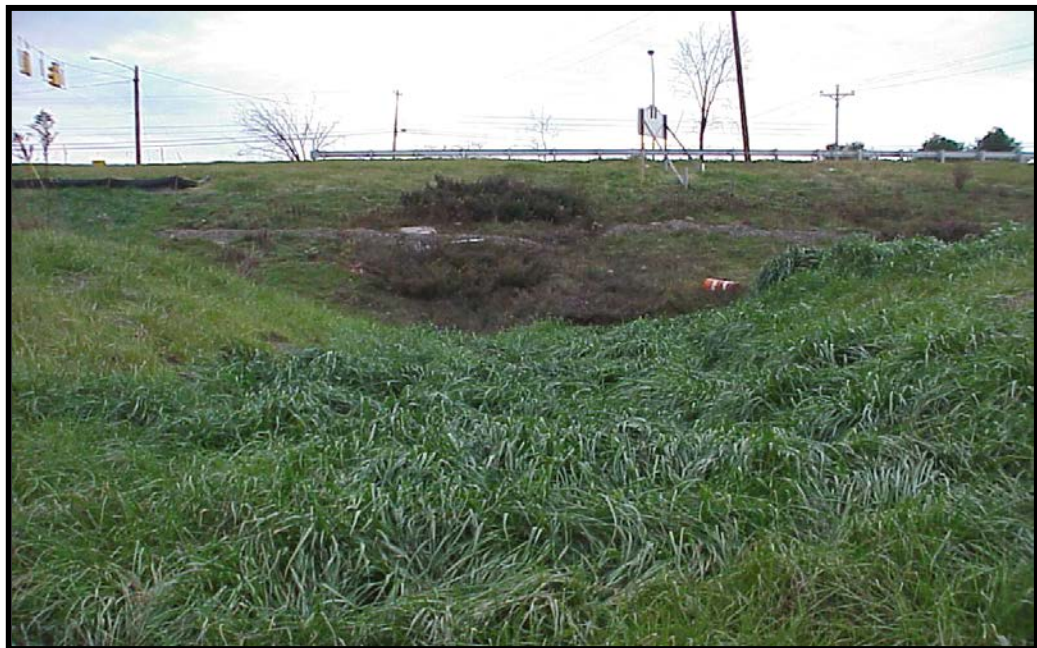
A WELL STABILIZED VEGETATED SWALE SHOWS LITTLE SIGNS OF EROSION VELOCITIES OR FLOWS. THIS SWALE ALSO FUNCTIONS AS A POND SPILLWAY
