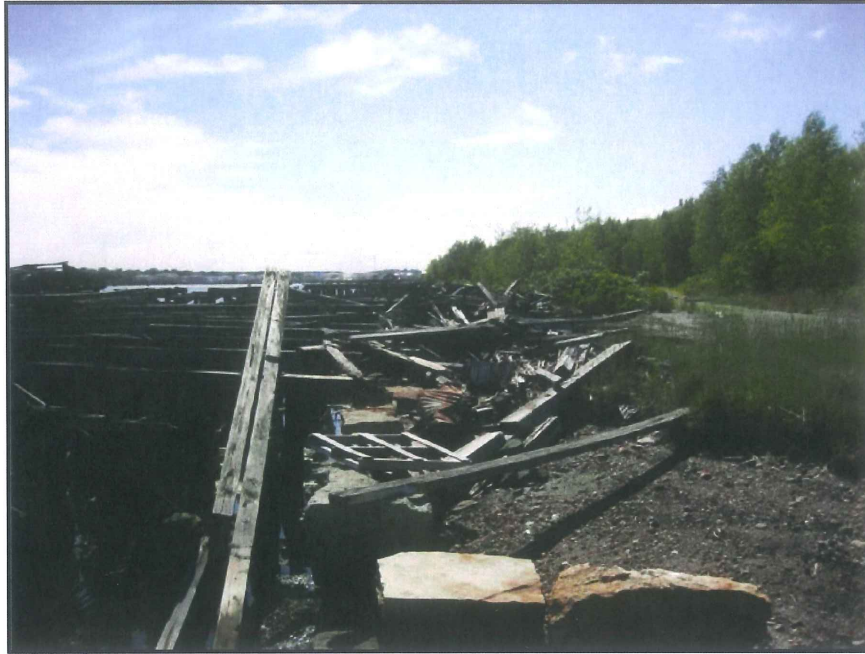
PHOTO 1 – Dilapidated Pier Remains
