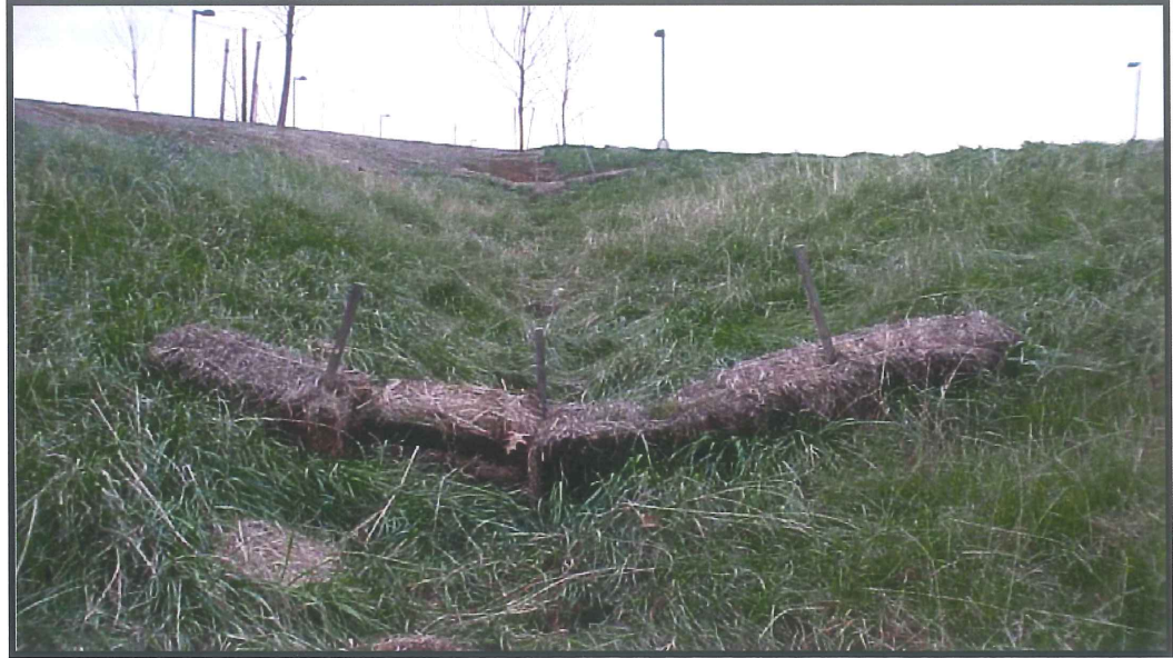
VEGETATED SWALE WITH HAY BALE CHECK DAM TO REDUCE VELOCITIES UNDER CONSTRUCTION
