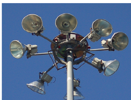
Fig. 9: High Mast Pole
