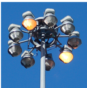
Fig. 8: High Mast Pole
