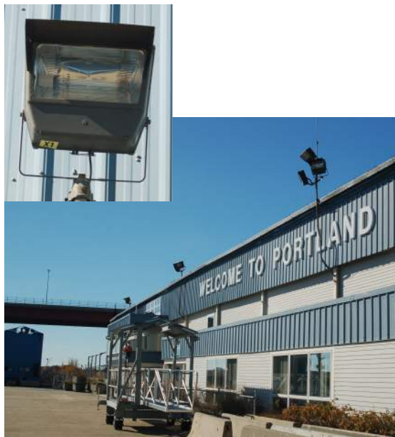
Fig. 2: Existing Building Mounted Pier Floodlights
