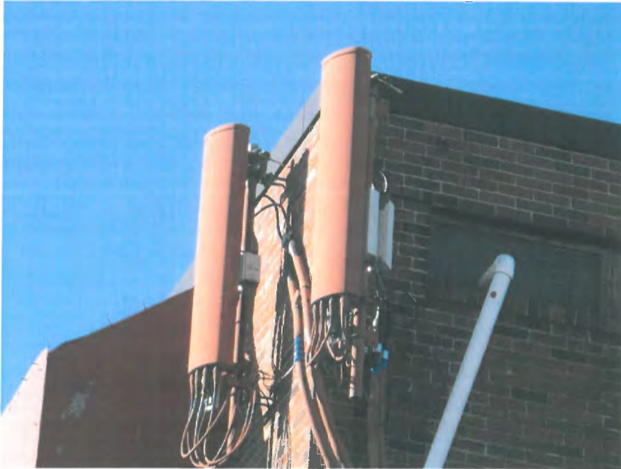
Photo 2: Sample photo illustrating the existing antenna mounted to penthouse
