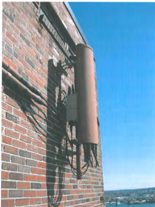
Photo 3: Sample photo illustrating the existing antenna mounted to the penthouse wall.
