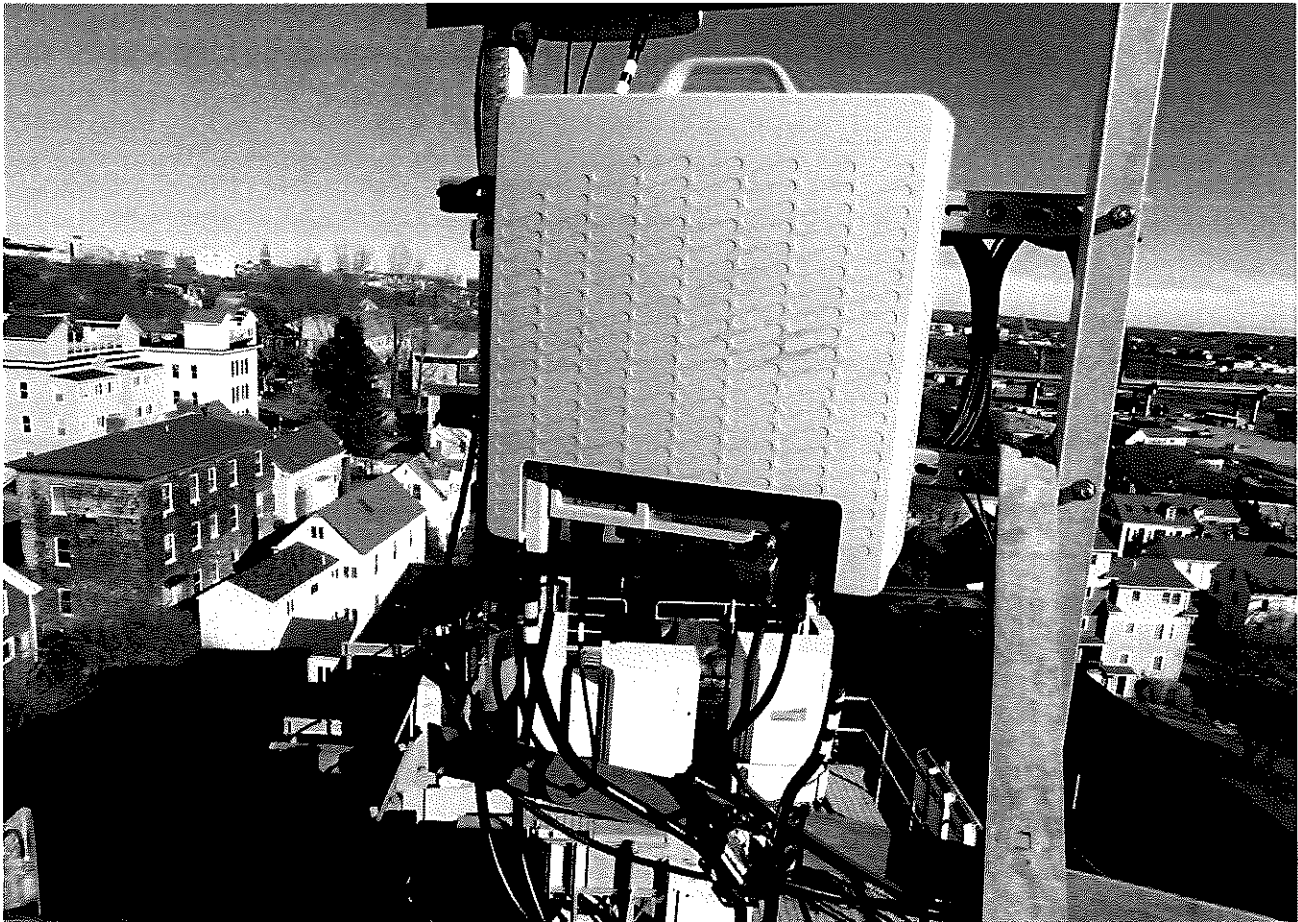
Close Up of RRU Mounted at Sector B
