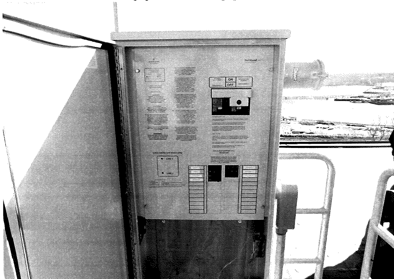
New PPC Mounted on New Equipment Frame
