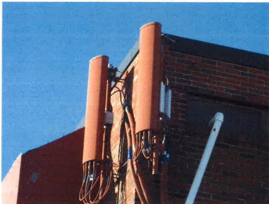
Photo 2: Sample photo illustrating the existing antennas mounted to the penthouse.
