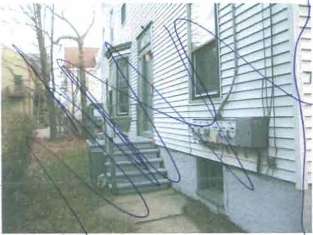
3) View of separate electric meters and side entrance 1 st floor
