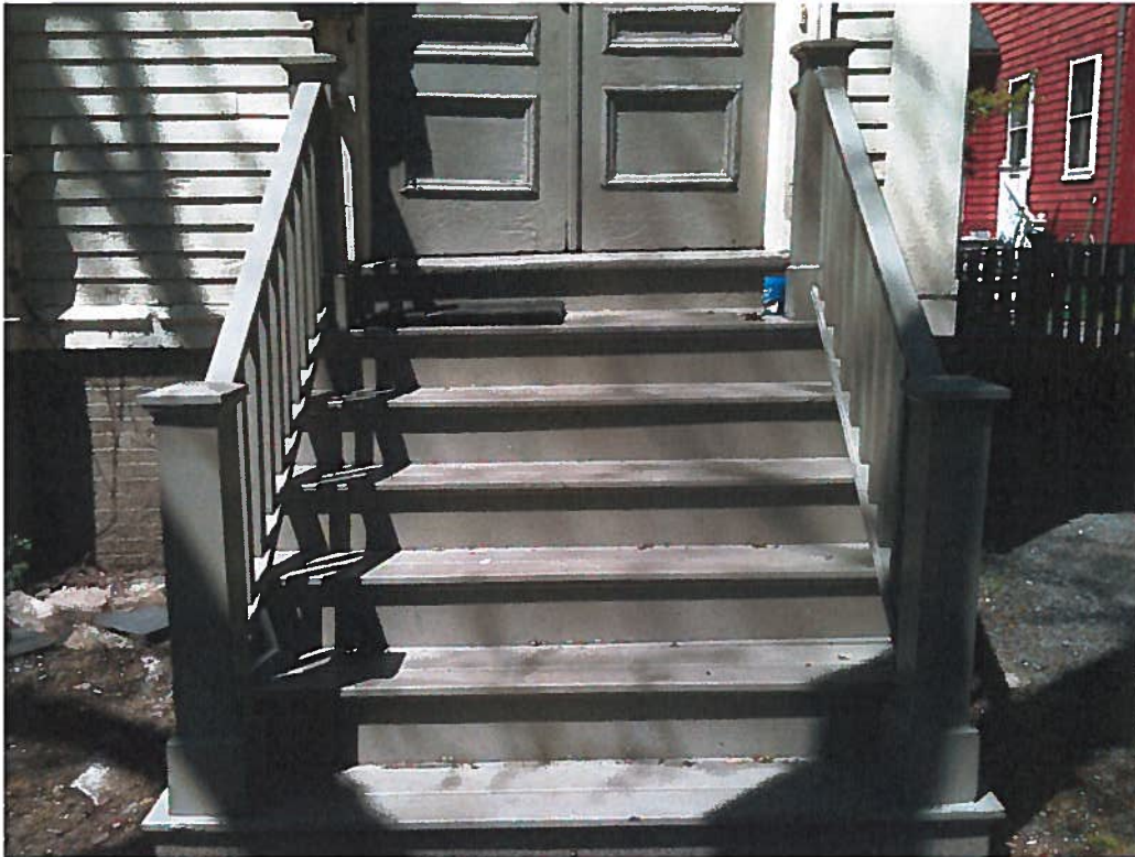
65 Spruce Street - Sample Finished Stair
