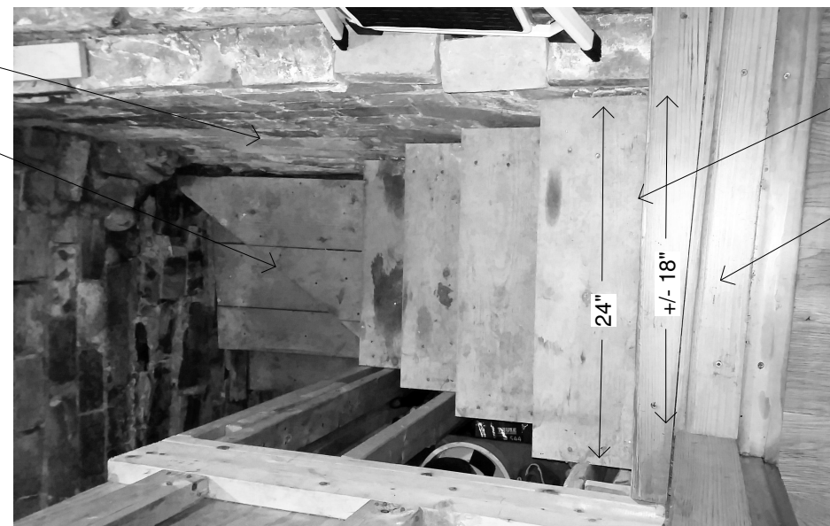
EXISTING NON COMPLIANT BASEMENT STAIR TO BE REMOVED
