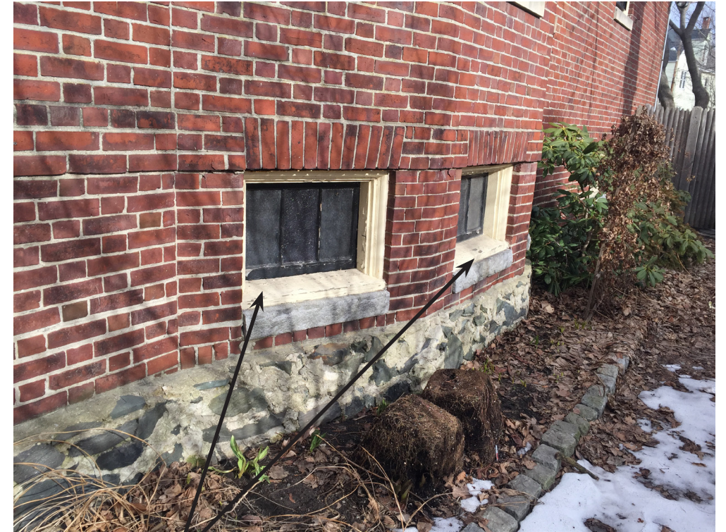
SIDE WINDOWS TO BE REPLACED
