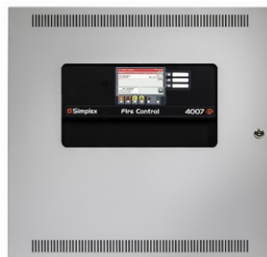
4007ES Fire Alarm Control Panel
