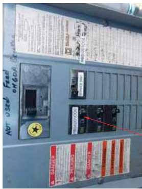
EXIST 60A-2P CIRCUIT BREAKER FOR EXIST. RES. 620T EQUIPMENT CABINET (UPGRADE TO 100A-2P)
