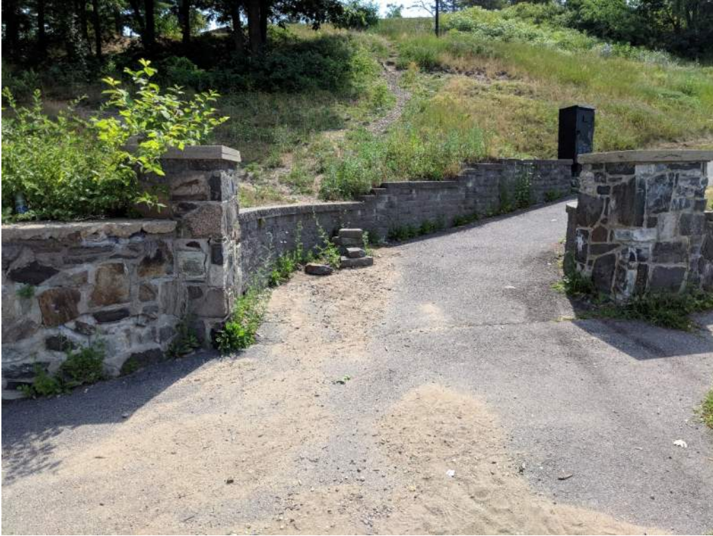
Photo 1: Erosion from retaining wall
